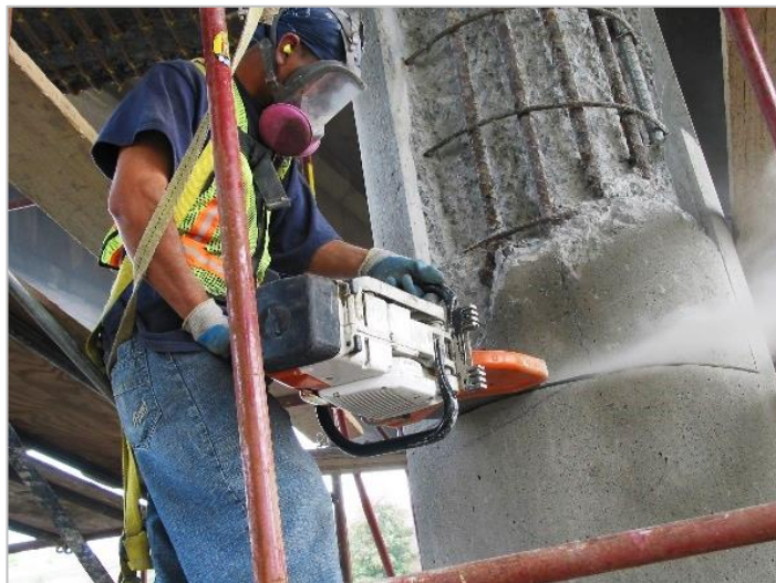
Worker generating respirable crystalline silica dust while cutting concrete bridge column
