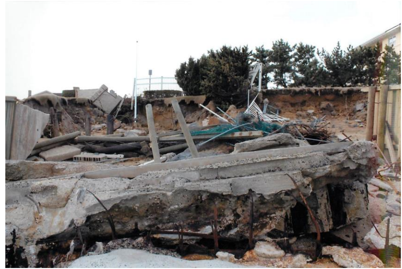
Figure 6: Damage to the end of Roseld Avenue, Looking West
