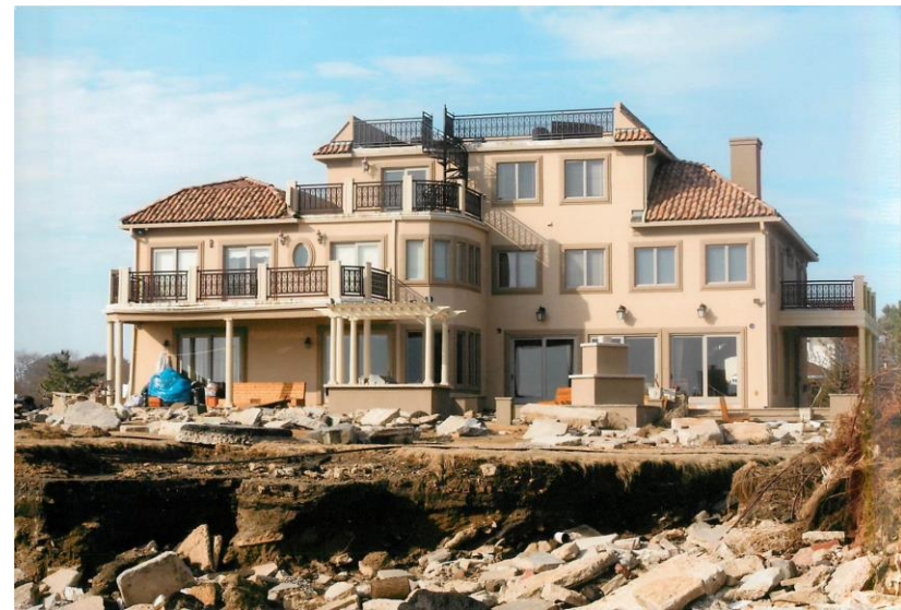
Figure 10: Debris and Erosion of the Shoreline at 10 Roosevelt Avenue.
