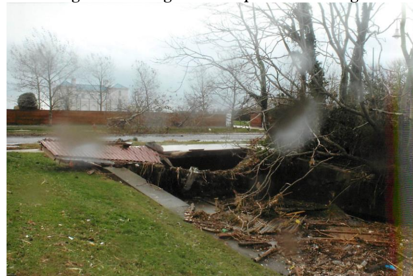
Figure 4: Damage at the Poplar Brook Bridge
