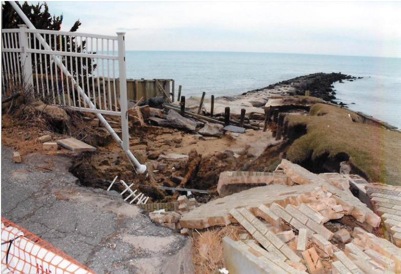
Figure 5: Damage to the end of Roseld Avenue, Looking East
