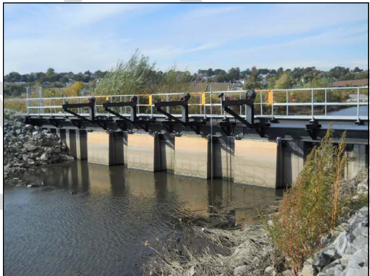
The Berry's Creek Tidal Gate has been repaired and upgraded to protect Teterboro Airport from daily tidal flood-
