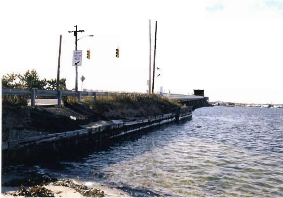
Photo 27: Herbert Street, east of Mantoloking Bridge facing southwest to Barnegat Bay.
