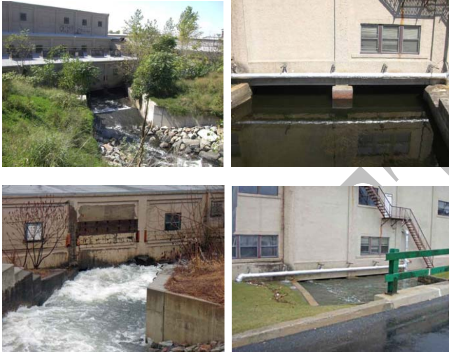
Old mill building across the Musconetcong River in Stanhope, low water (top) and high water (bottom)
