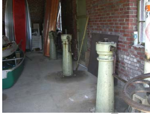
Hand cranks control sluice gates and fountain
