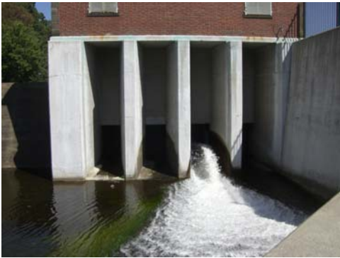
Lake Hopatcong sluice gates
