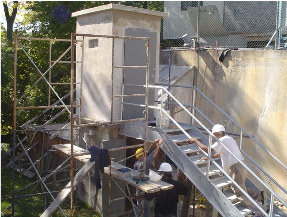
Photo 2: View of the ongoing work to flood harden the USGS gage at the Delaware River Trenton (01463500). A second story has been added to the gatehouse.
