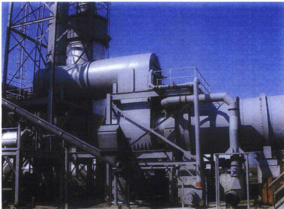
Figure 2. The Cement-Lock Demonstration Plant from the South
