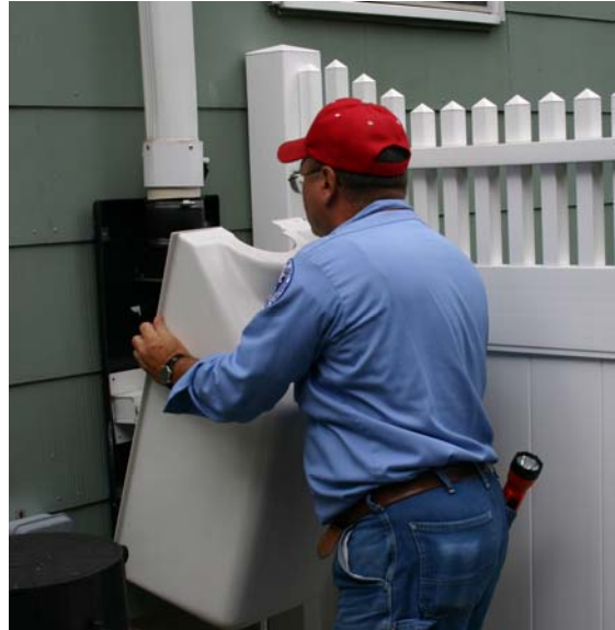
Inspection of SSD fan and weatherproof cover
