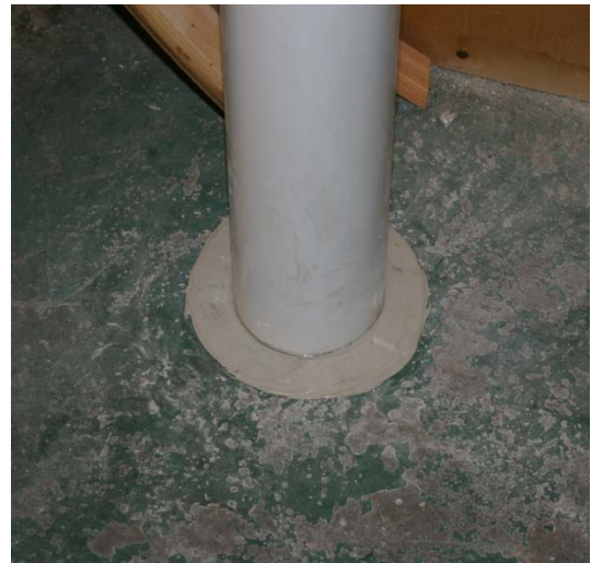
Proper sealing around suction point
