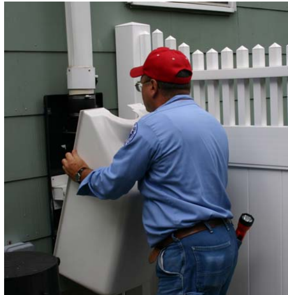
Inspection of SSD fan and weatherproof cover
