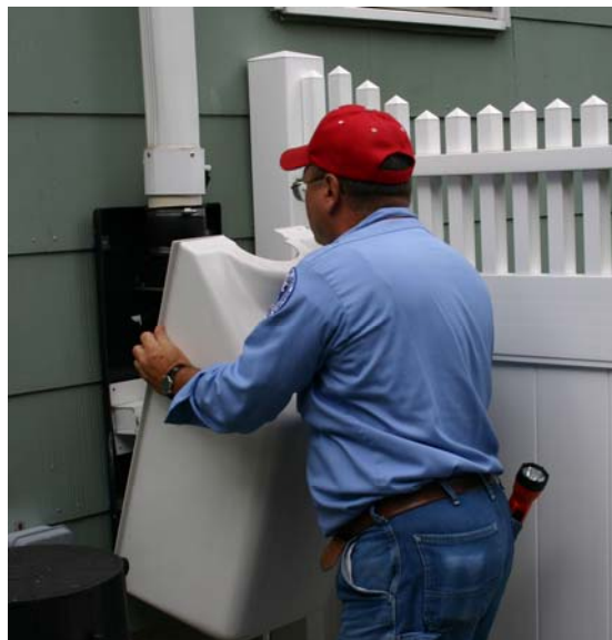
Figure 6-1. Inspection of SSD fan and weatherproof cover
