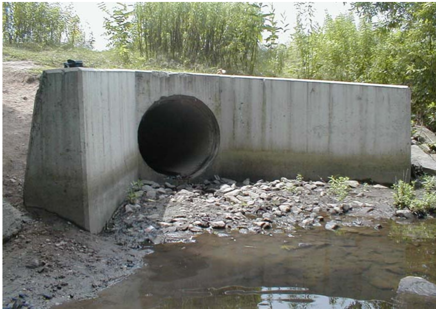
Figure A - Stormwater outfall discharging directly into Pascack River at upstream end of sampled reach at site FIBI059.
