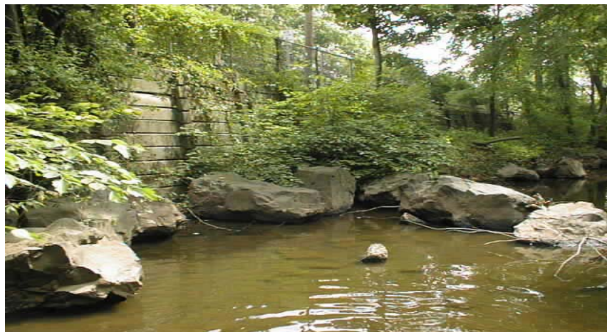
Figure C – Retaining wall and displaced rock rip-rap.
