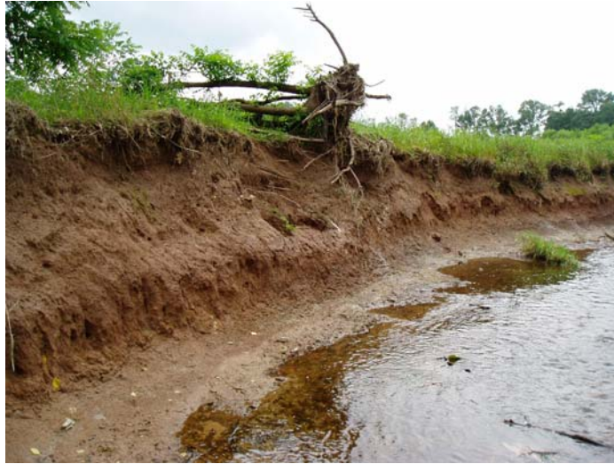
Figure 7. Severe bank erosion on the Neshanic River
