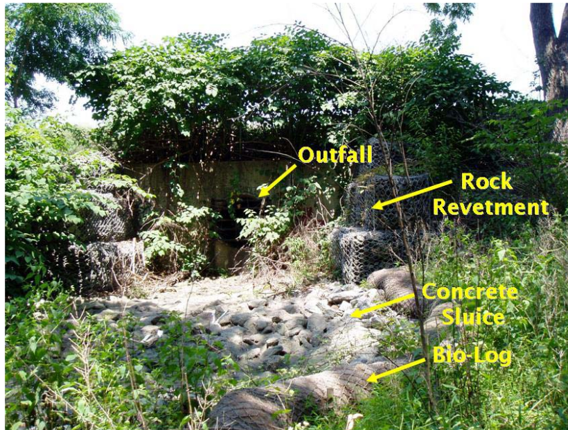
Figure 9. Erosion control structures around a storm sewer outfall on the Passaic River.
