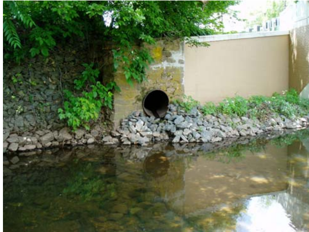
Figure 17. Storm sewer outfall near end of stretch on Peters Brook.
