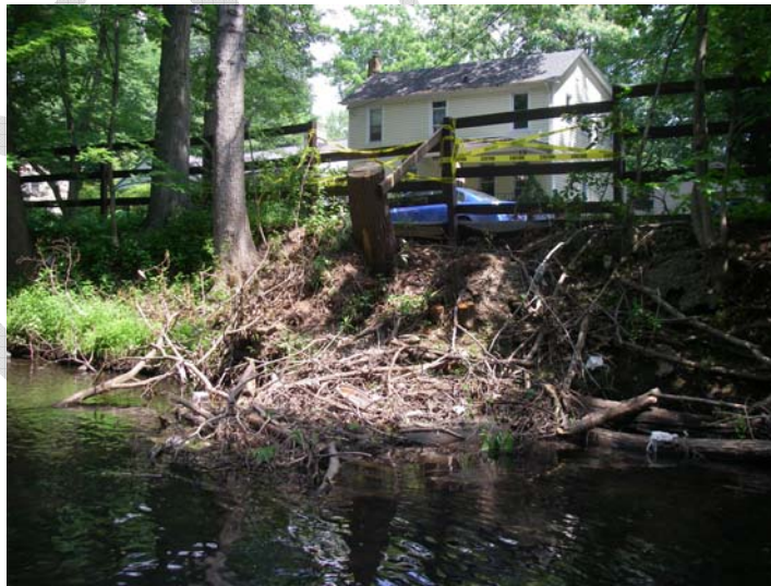
Figure 10. Severe bank erosion along Rahway River.
