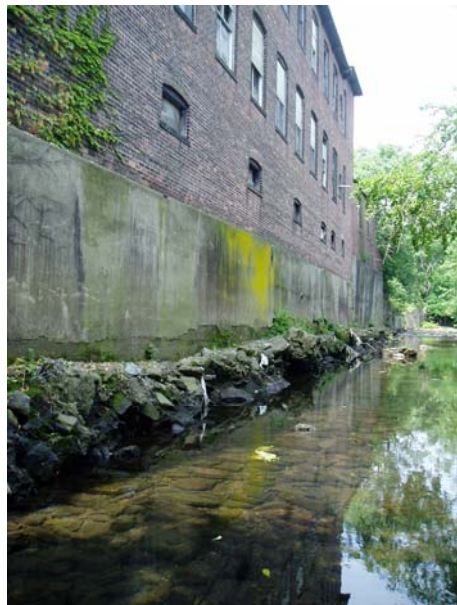
Figure 19. Factory with numerous outfalls and concrete armored bank along Second River.
