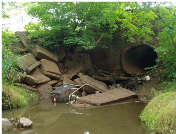
Figure 14. Debris, concrete slabs, and storm sewer outfall on Royce Brook.
