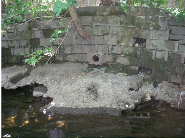
Figure 9. Concrete debris in Van Saun Mill Brook.
