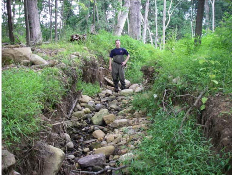
Figure 22. Channel scouring at storm water detention basin outlet.
