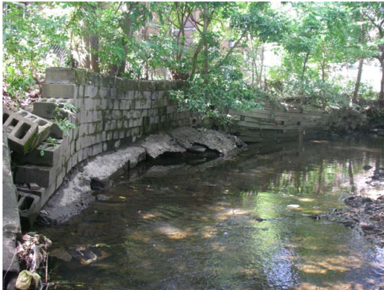
Figure 8. Failing retaining walls along Van Saun Mill Brook.
