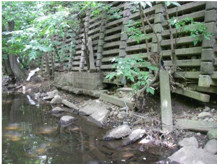
Figure 12. Failing retaining wall on Mahwah Brook.
