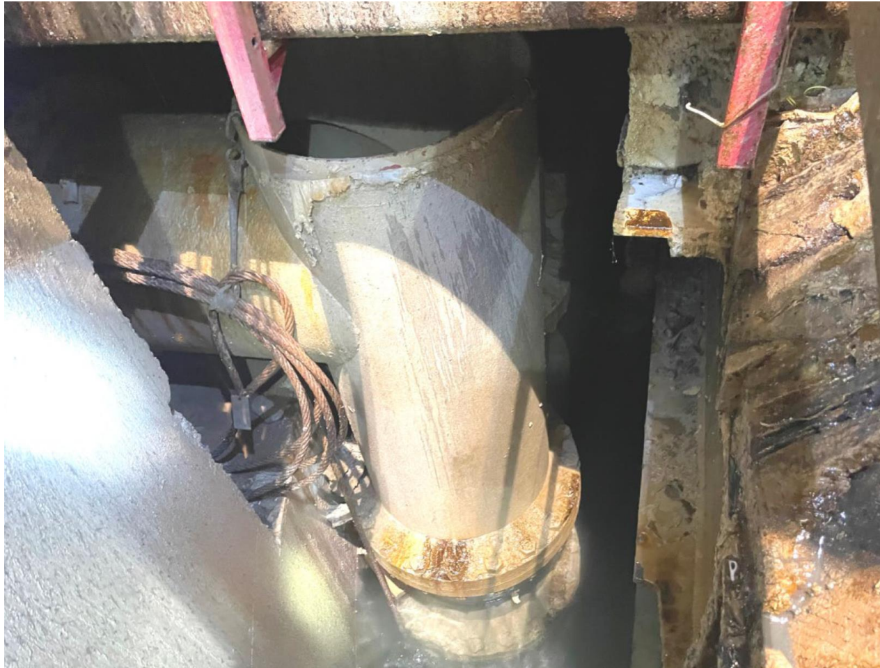
Baffle Drop Pipe
