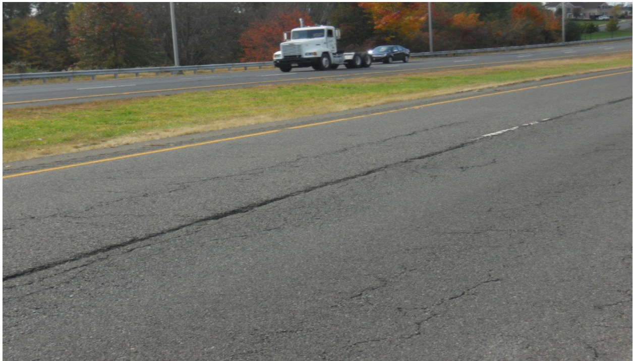
WB MP: 26.69- H-Longitudinal cracking between lanes; M-Fatigue cracking.
