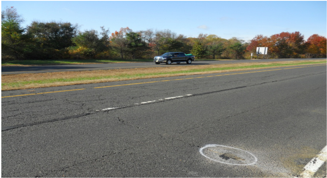
WB MP: 25.04- Fatigue cracking in Lane 1; Transverse & longitudinal cracking; H-longitudinal cracking between lanes.
