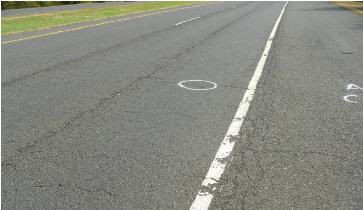
EB MP: 24.50- M-Longitudinal & transverse cracking in Lane & Outside Shoulder.
