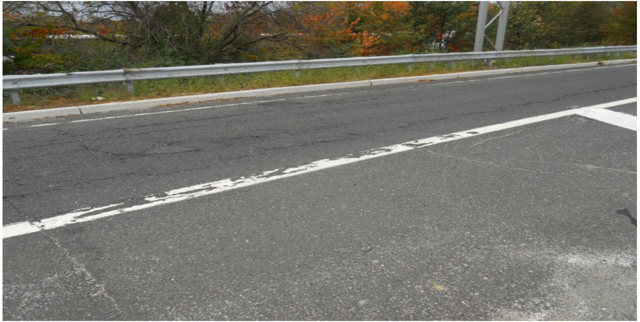
Ramp MP: 27.54- Fatigue cracking.
