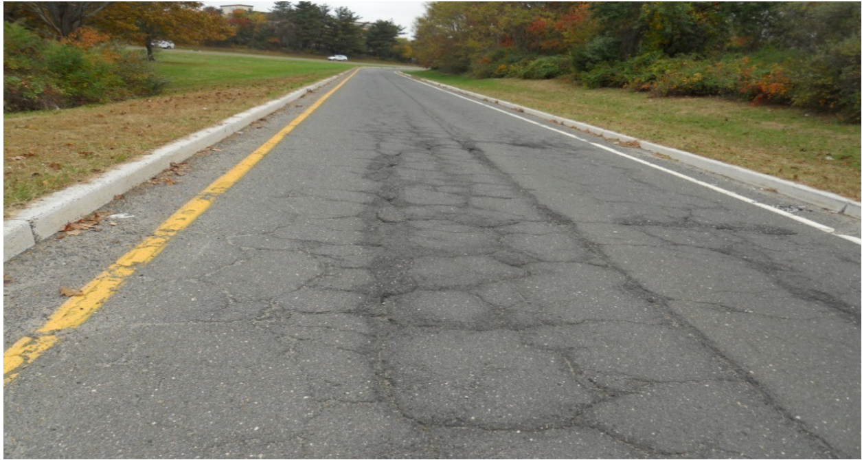
Ramp MP: 26.59- Block cracking.
