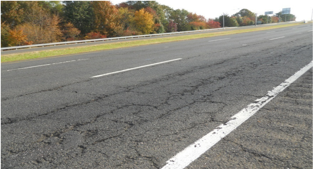
EB MP: 28.55- M-Block & fatigue cracking; M-Longitudinal cracking between lanes.
