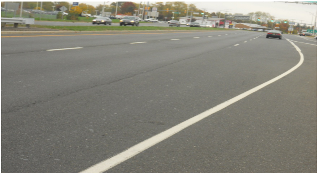
Rt. 9 Underpass MP: 27.54- L-Longitudinal cracking between lanes.
