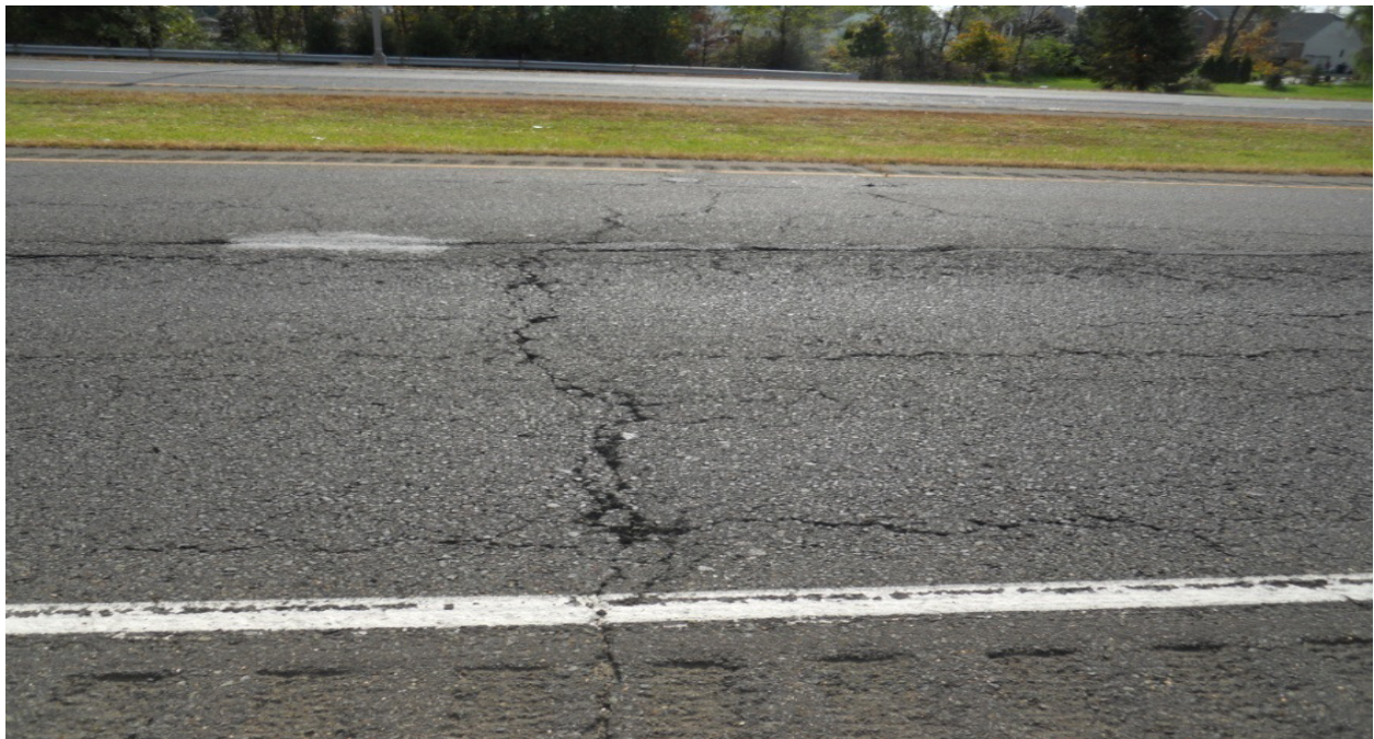
WB MP: 26.43- H-Transverse cracking & L-longitudinal cracking; H-Longitudinal cracking with patching between lanes.
