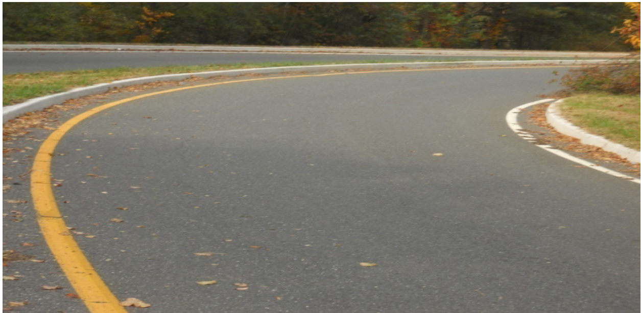
Ramp MP: 25.68- Minimal distress
