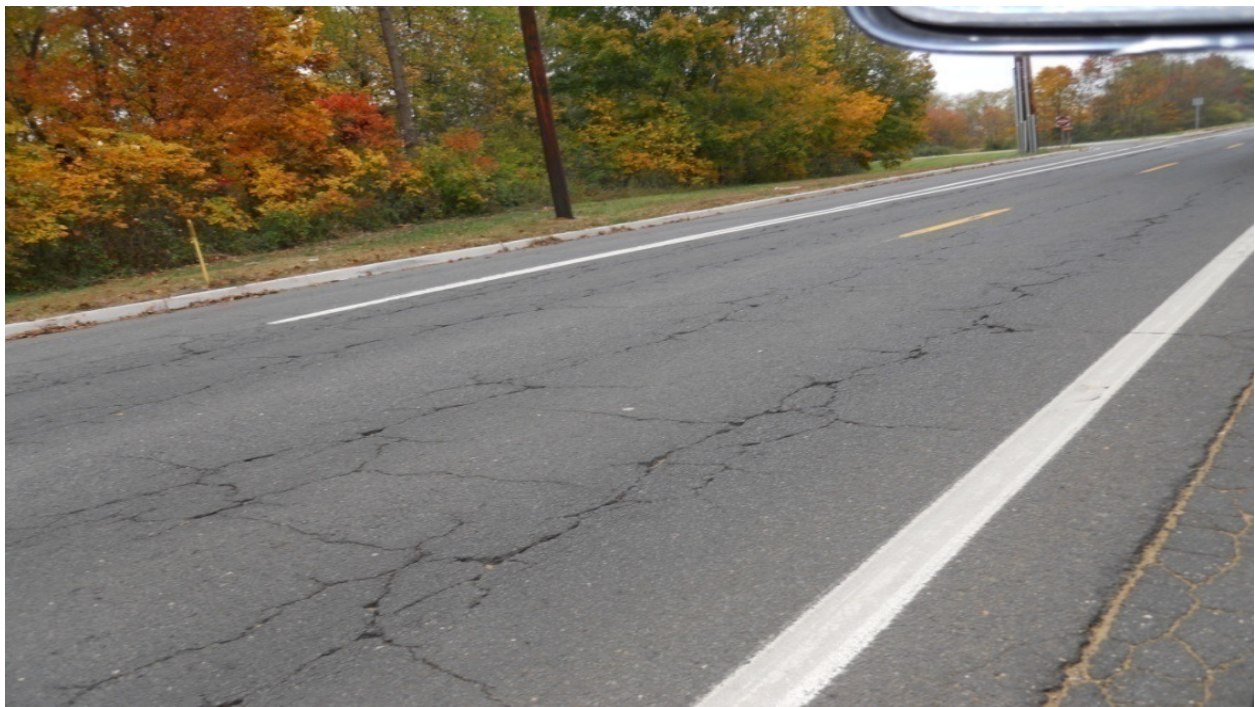
Wemrock Road Overpass MP: 25.68- Fatigue & block cracking.
