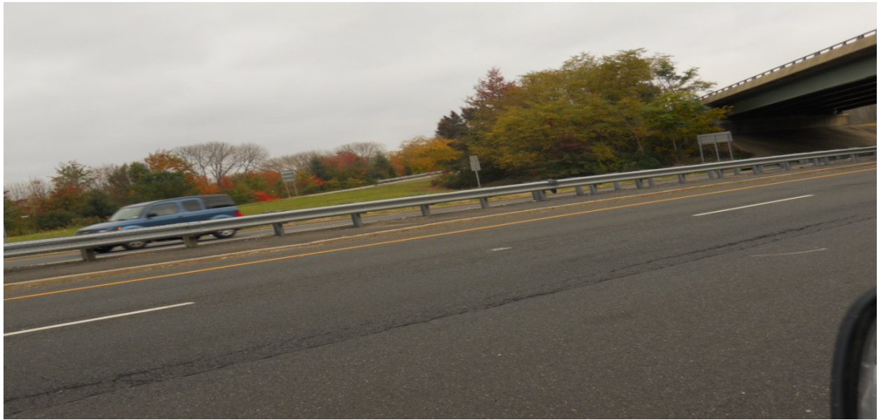
Rt. 9 MP: 27.54- M-Longitudinal cracking between lanes.
