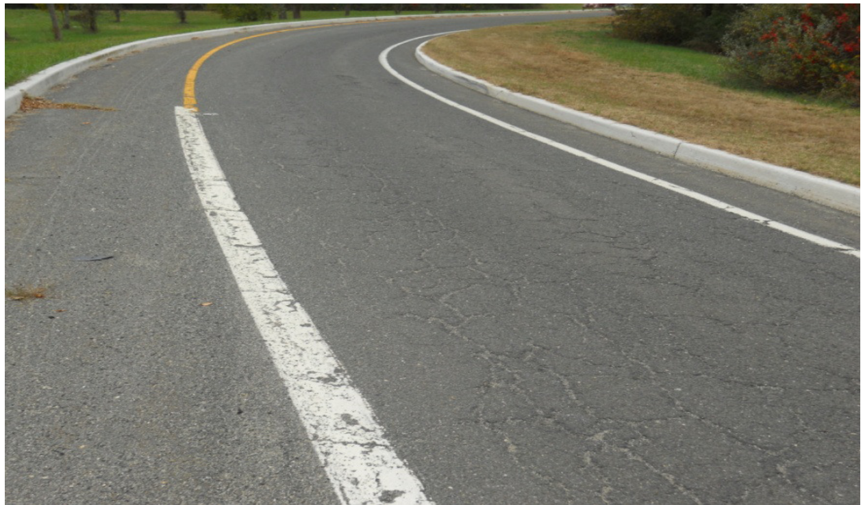
Ramp MP: 25.68- Fatigue cracking.
