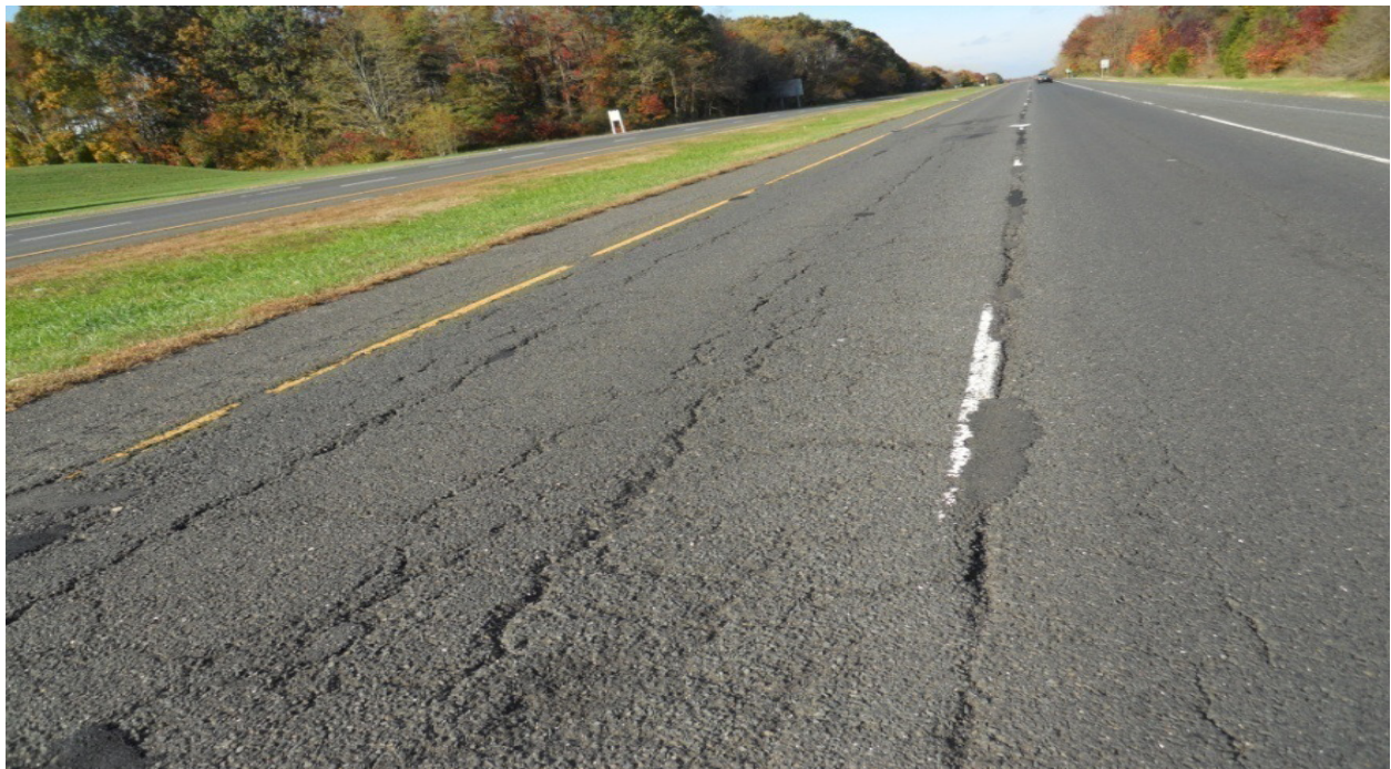
WB MP: 25.47- Fatigue cracking, rutting, & H-longitudinal cracking with patching between lanes.
