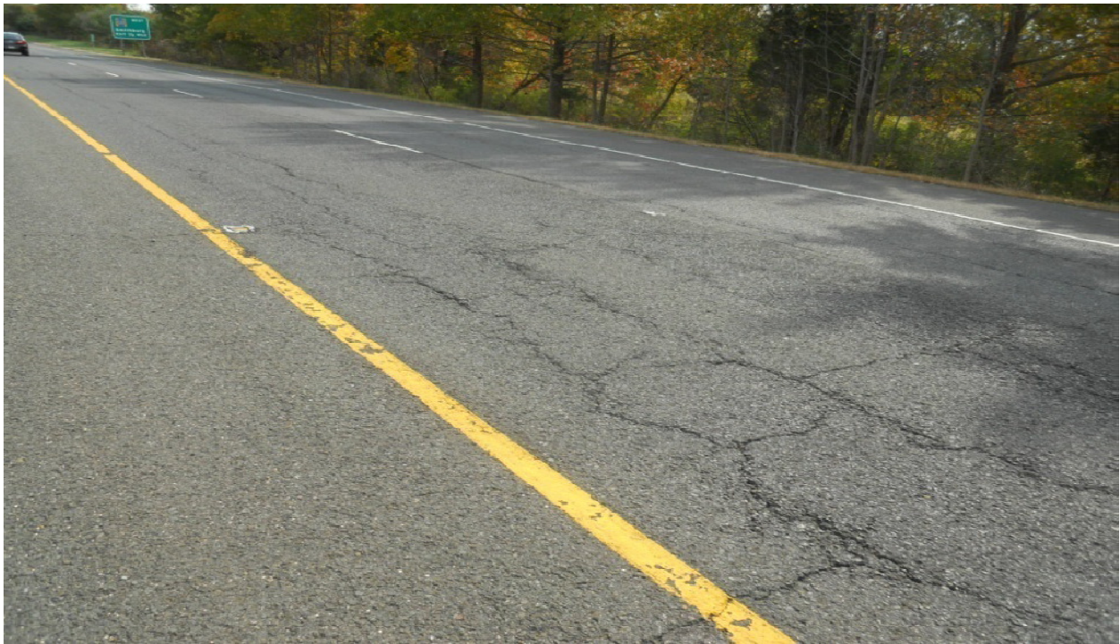
EB MP: 24.92- M-Block cracking
