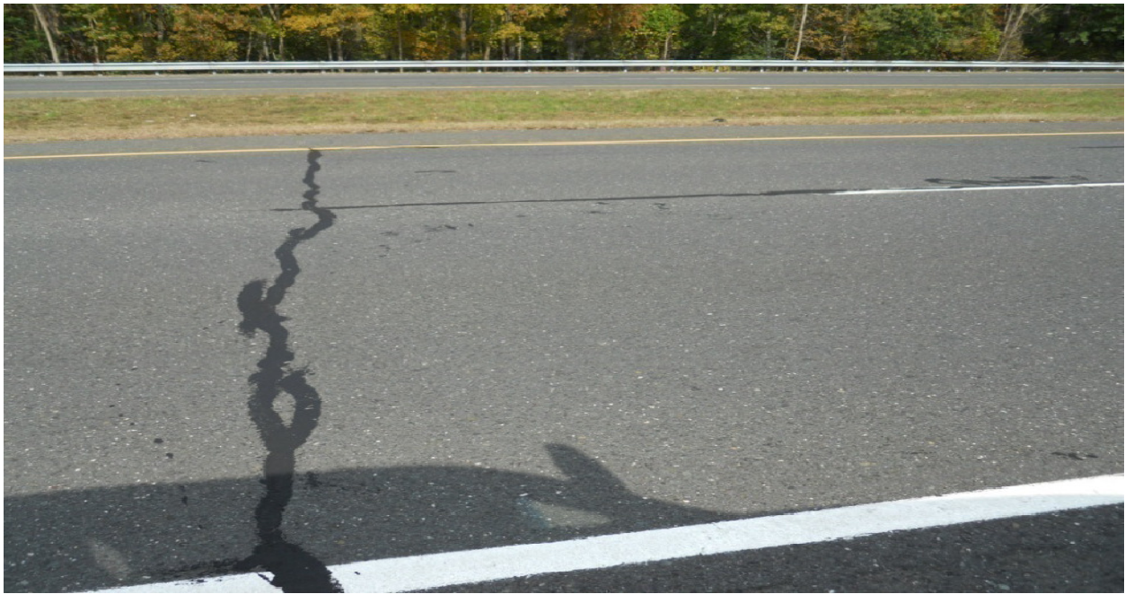
EB MP: 25.87- Sealed longitudinal & transverse cracking.
