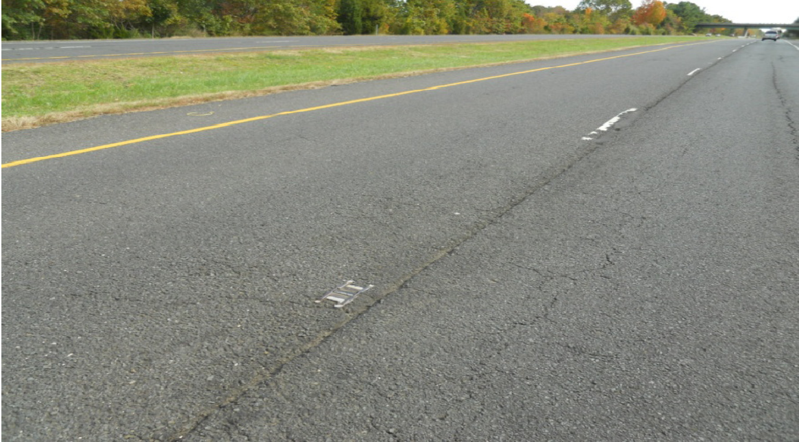
EB MP: 24.51 M-Longitudinal cracking between lanes; L-Fatigue cracking
