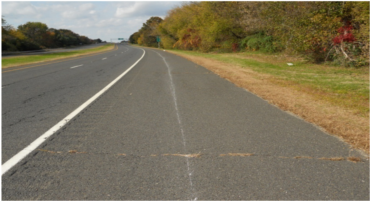
WB MP: 27.42- M-Transverse cracking.
