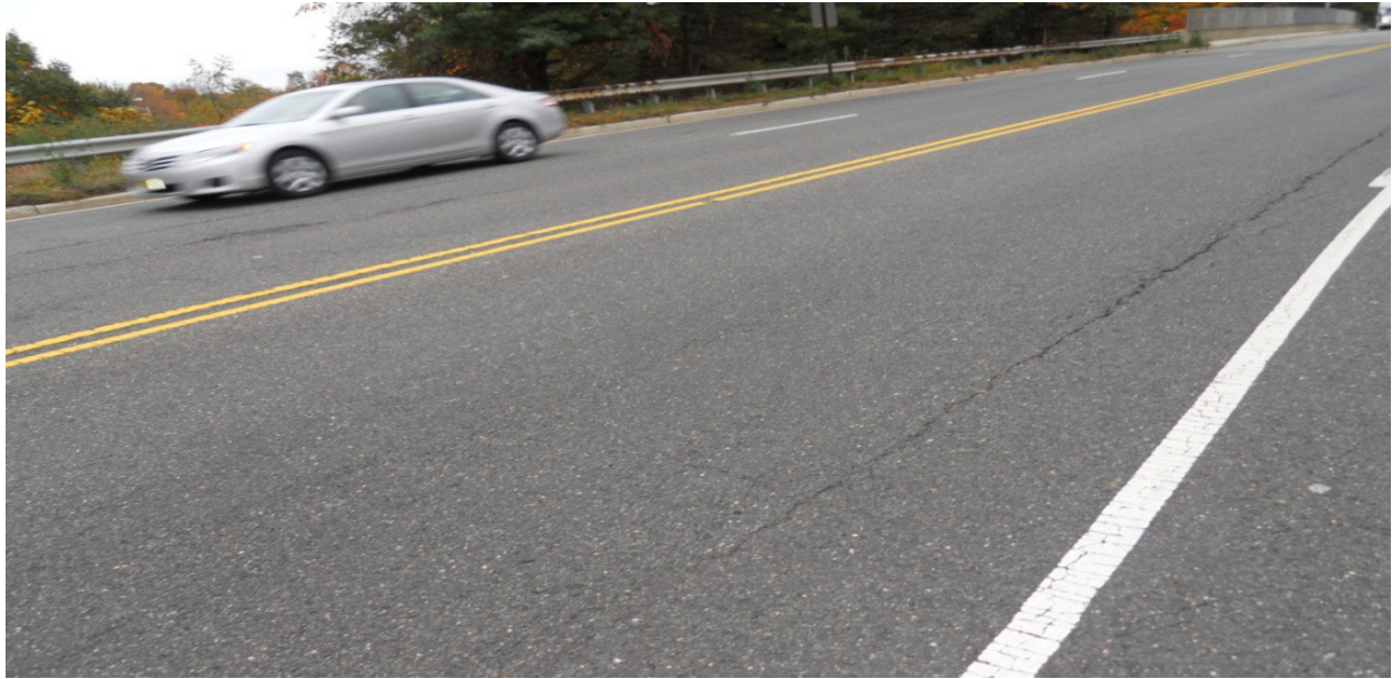
CR-537 Overpass MP: 26.59 - L-longitudinal cracking
