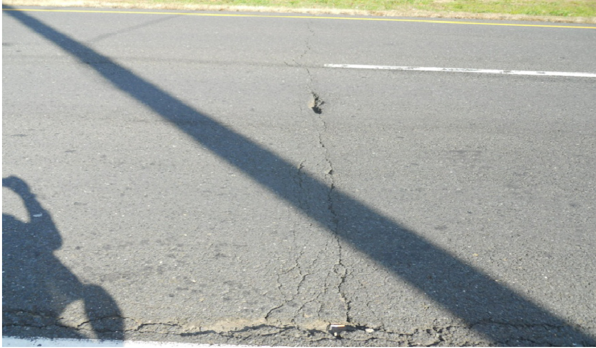
EB MP: 24.21- M/H-Transverse & longitudinal reflection cracking.
