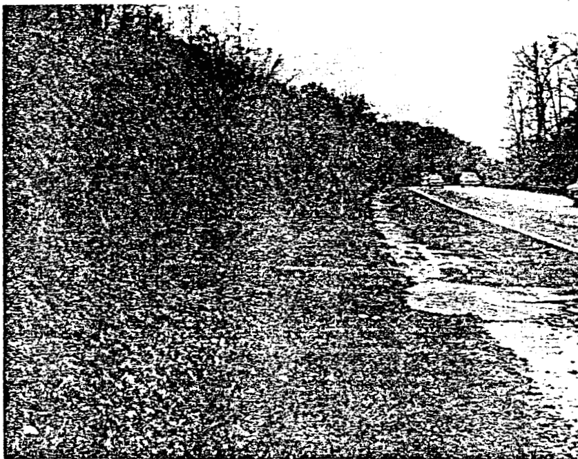
Figure 4: Route 287 northbound @ M.P. 26 Another example of runoff drainage in a cut.
