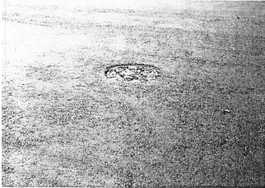
PHOTO 13 POOR RESET - POOR RIDEABILITY
