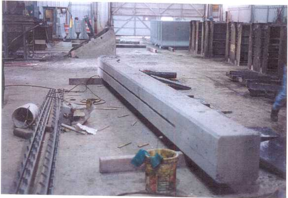
Fig. 6. Concrete post - 24 ft. long with channel for T bolts cast in. Note: Halfan Channel on left.
