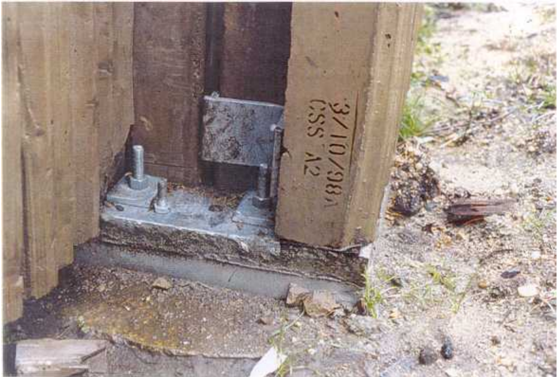
Fig. 45 Post base plate set on anchor bolts with grout below. Note anchor bolt and panel angle interference.
