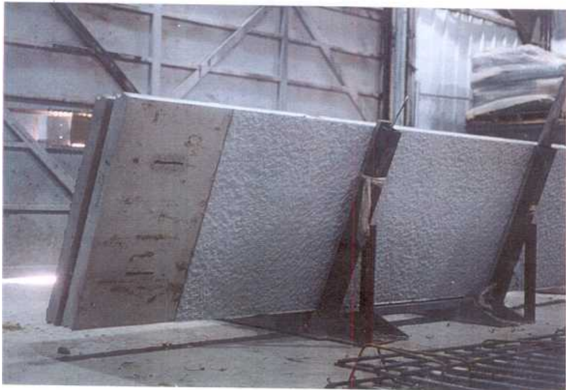
Fig. 2 Bush hammer (highway side) 4 ft. panel with smooth end treatments which rest against the posts.
