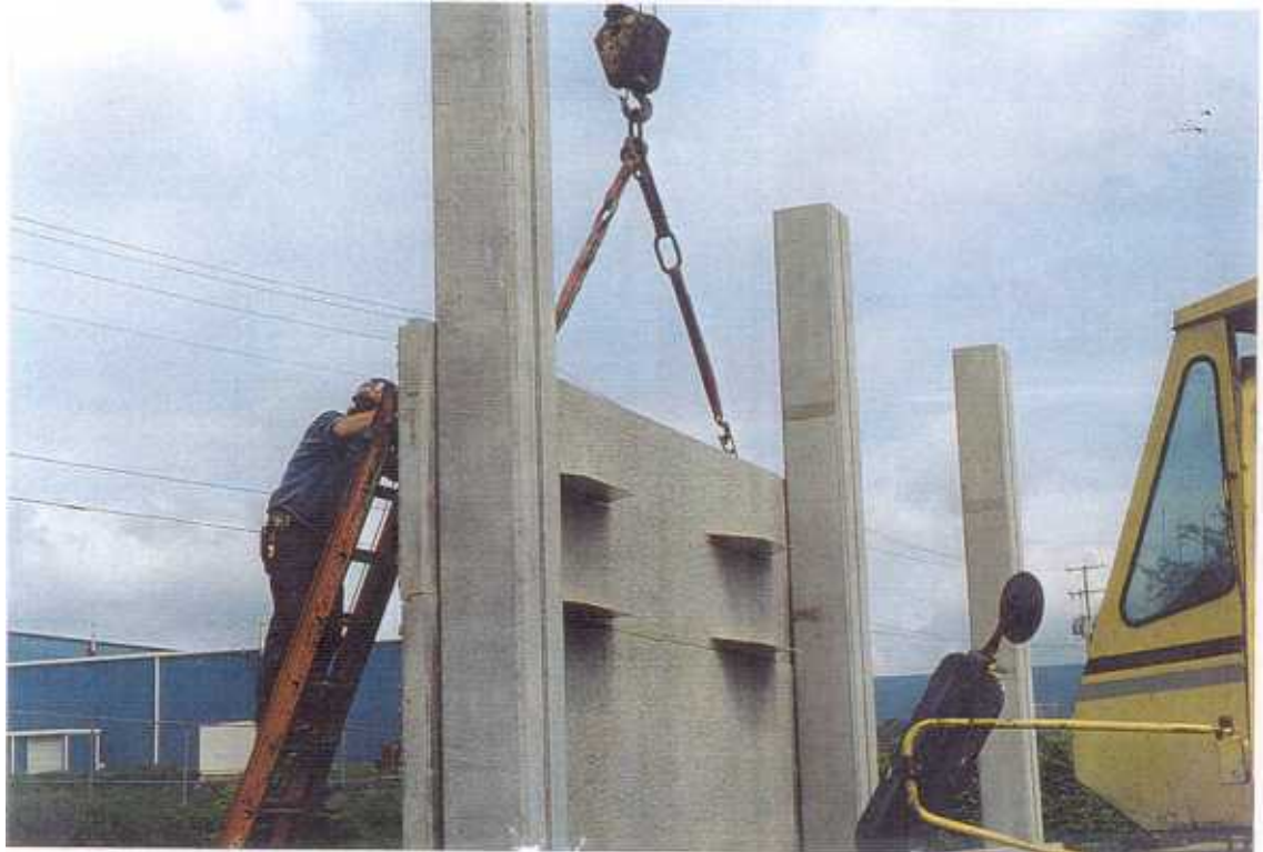
Fig. 16 Panel Fig. 15 being bolted from the residential side with the bush hammer side to the post.
