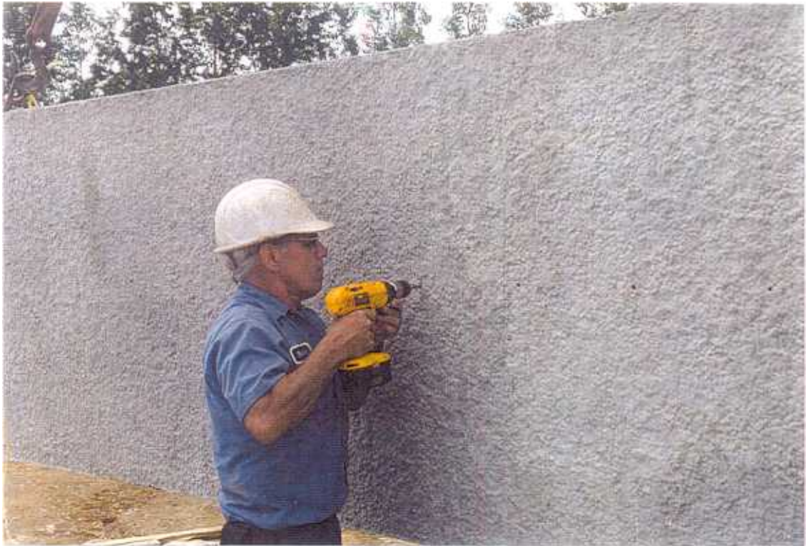
Fig. 13 Grout filled plastic anchors needed tapping
