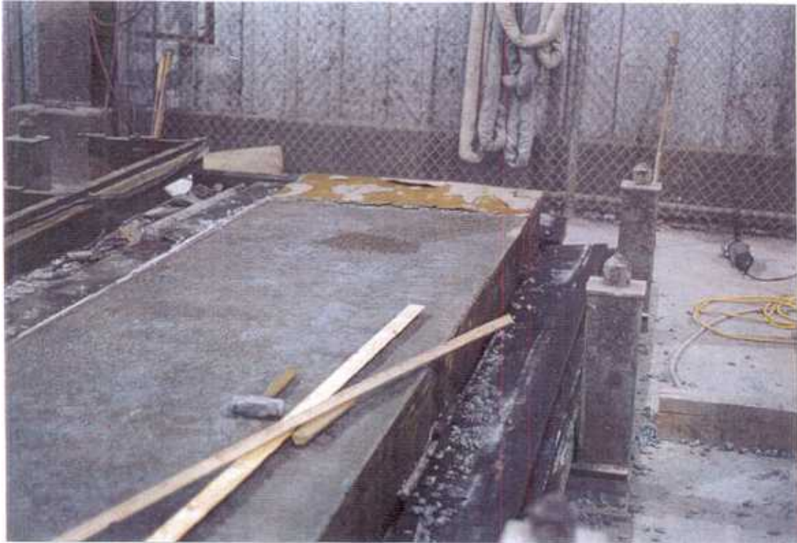
Fig. 1 Bush hammer (highway side) form liner at bottom of horizontal form at CSS.
