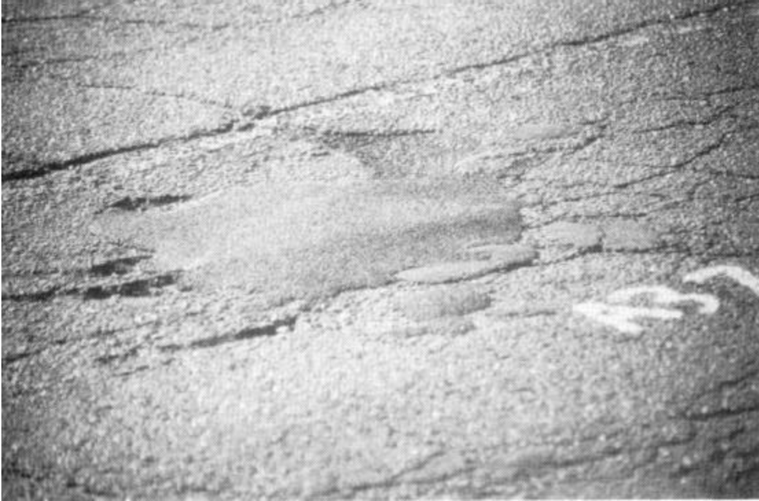
Figure 3. Edge Disintegration Distress (3)
