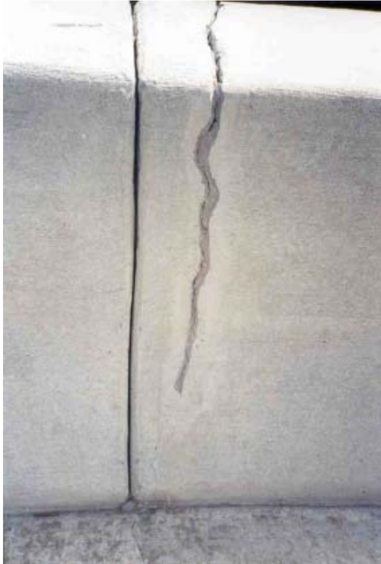
Figure 94. Crack on deck and parapet (Bridge No. 0173-151).
