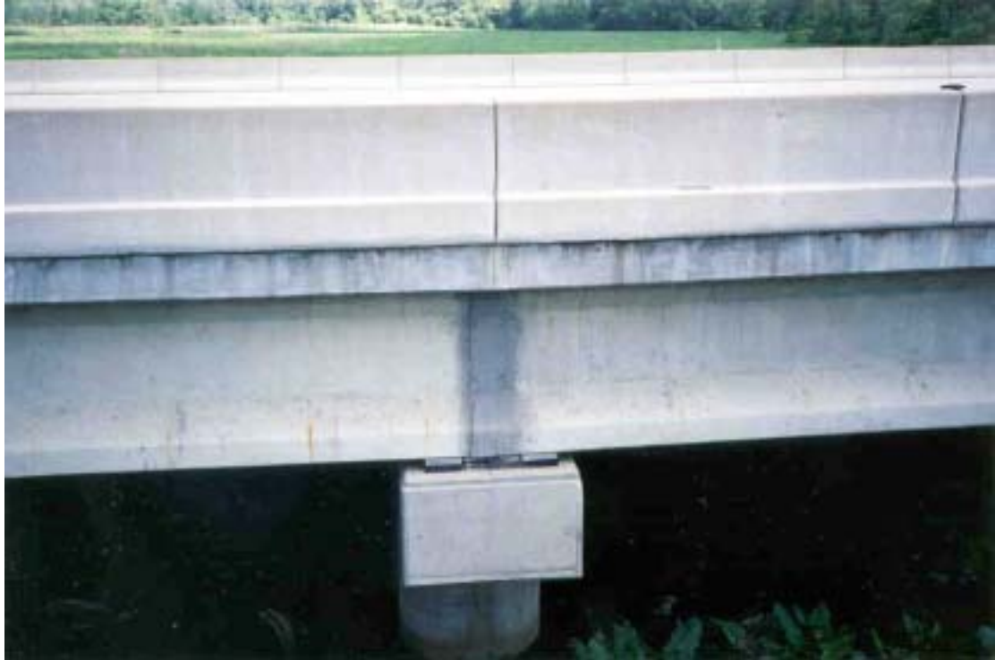
Figure 97. Cracked continuity joint (Bridge No. 1130-152).
