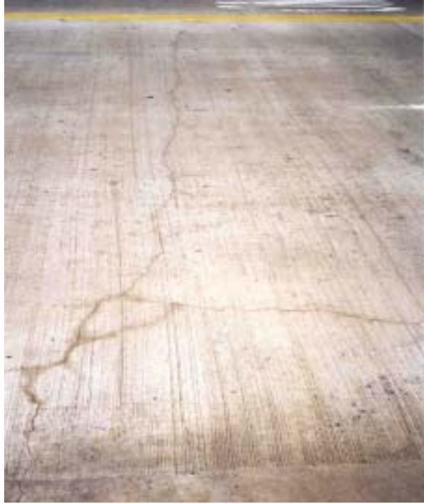
Figure 100. Transverse cracks on the deck (Bridge No.1130-153).
