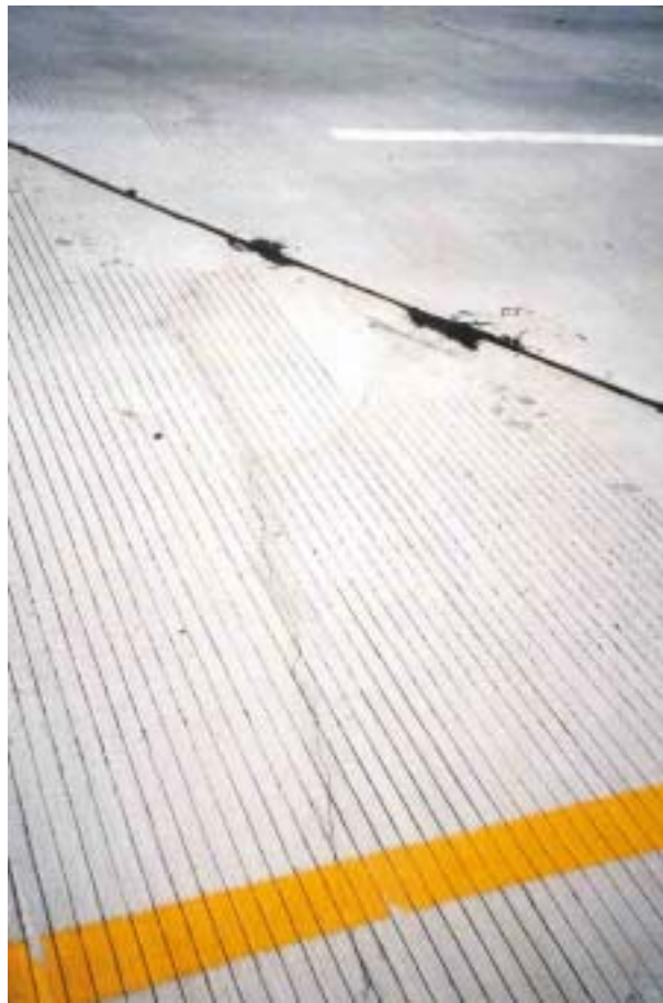
Figure 104. Close view of a crack (Bridge No. 1143-166).
