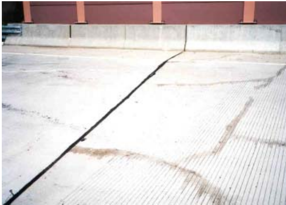
Figure 107. Transverse cracks on bridge deck (Bridge No. 1143-169).
