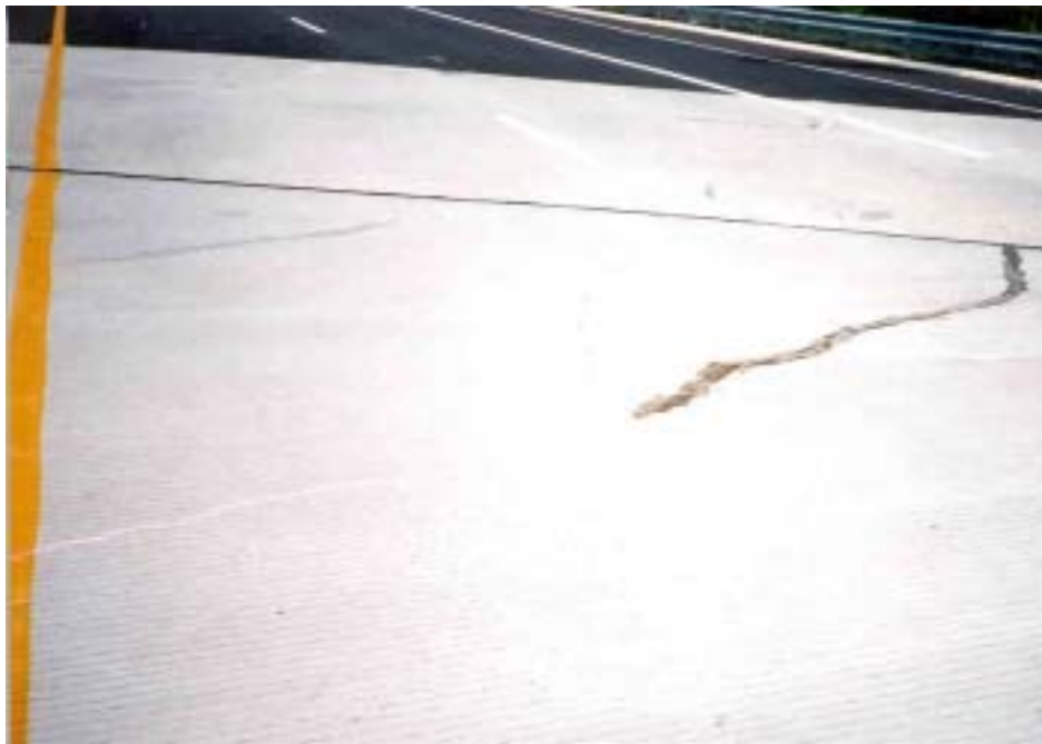
Figure 110. Cracks on the deck (Bridge No.1143-171).
