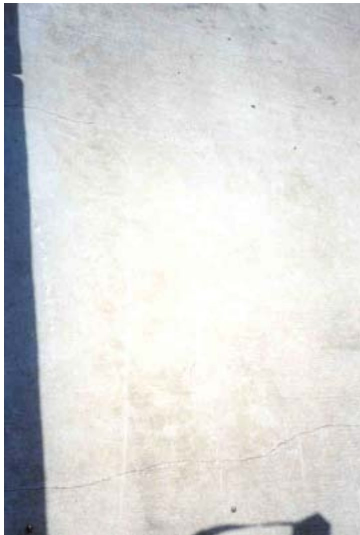
Figure 90. Crack on the deck (Bridge No 0713-151).
