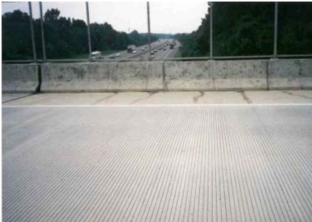
Figure 16. Rt. 133 bridge deck crack.
