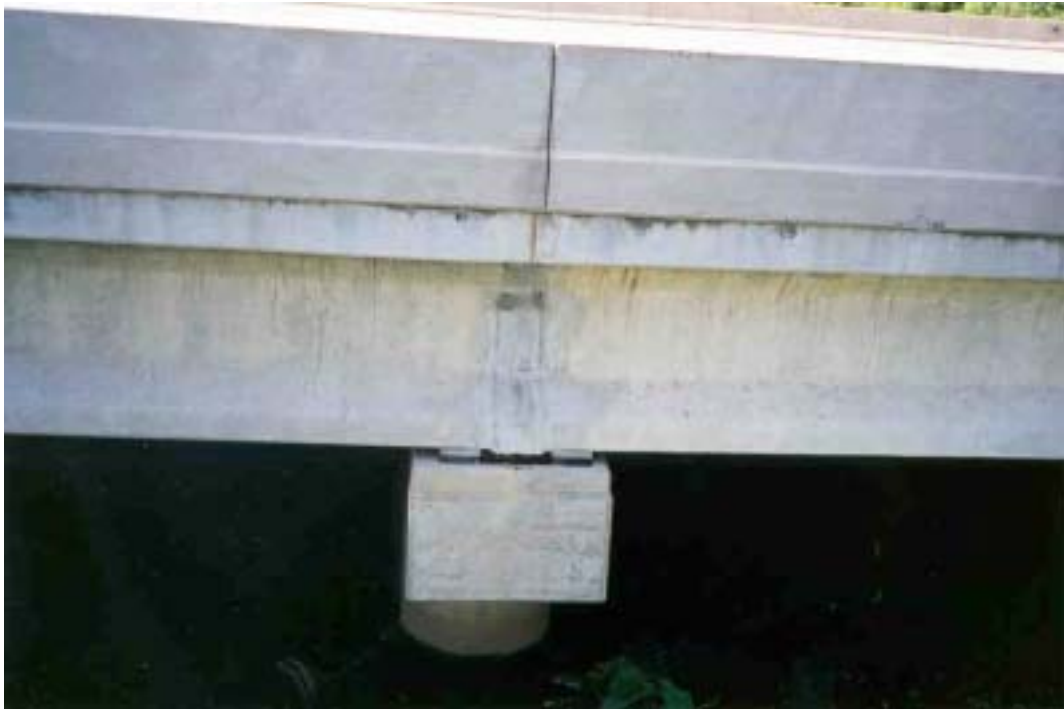
Figure 101. Un-cracked continuity joint (Bridge No.1130-153).
