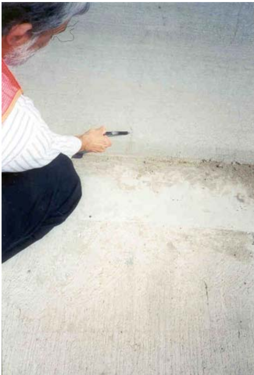
Figure 93. Crack extending into the parapet (Bridge No. 0713-151).
