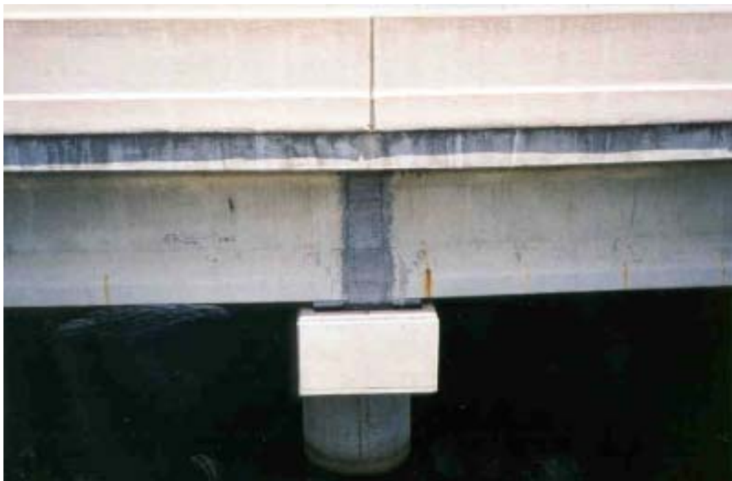
Figure 98. Another cracked continuity joint (Bridge No.1130-152).
