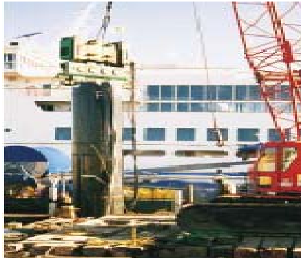
Figure A33. Installation of a Composite Monopile at Cape May, New Jersey
