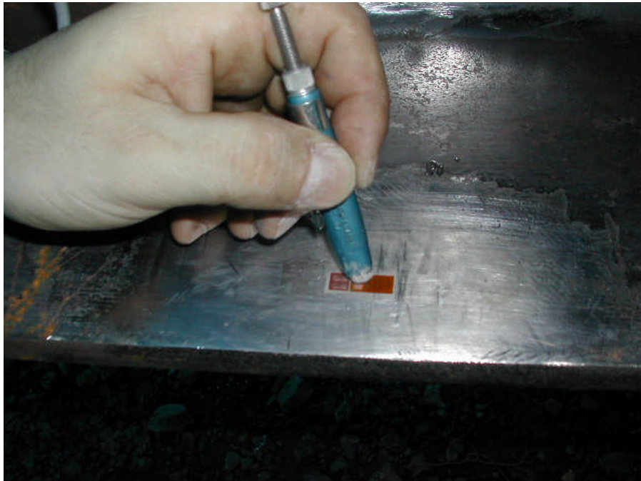
Figure 32. Preparing the surface for welding by removing any oxidation from the gage
