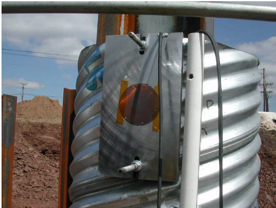
Figure 18. Installation of soil pressure cell on the exterior surface of galvanized-steel sleeve
