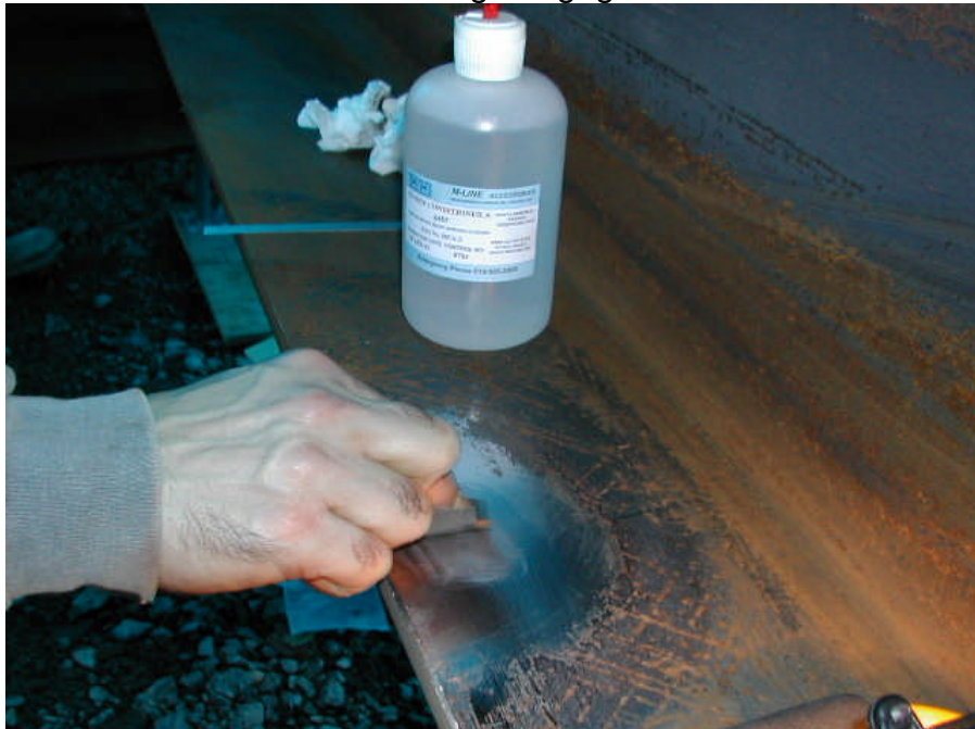
Figure 20. Grinding the surface with sand paper #100 at the location of installing the gage
