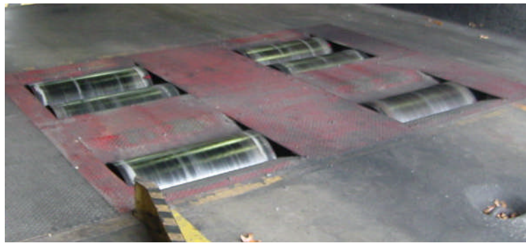
Figure 35: Water brake dynamometer installed in ground
