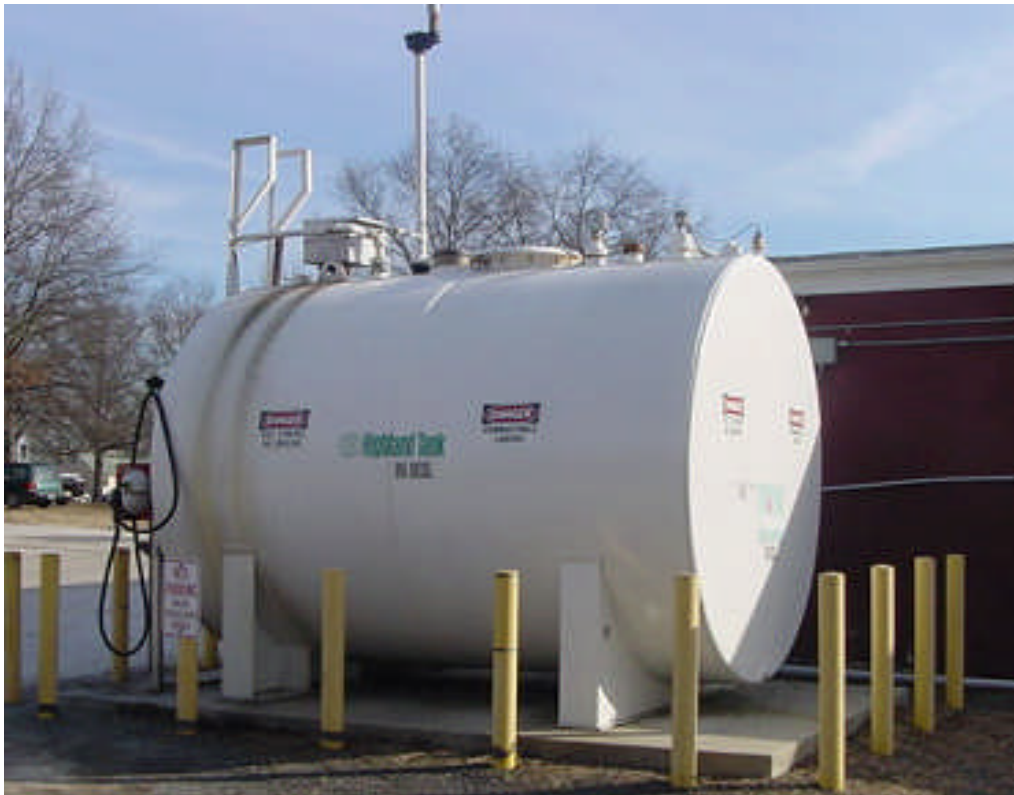
Figure 63: Medford biodiesel storage tank
