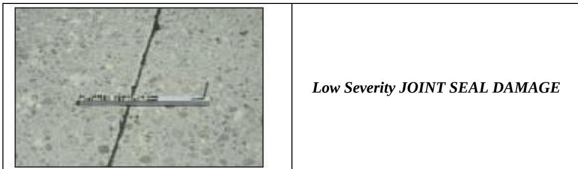
Figure 20. JOINT SEAL DAMAGE
