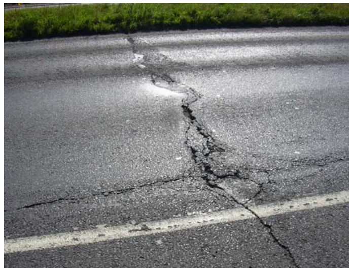
Figure 1 – Reflective Cracking of Flexible (Asphalt) Overlays on Rigid (PCC) Pavements
