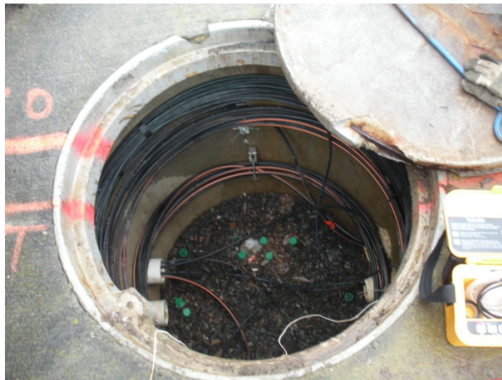
Figure 2: View of manhole with cover removed. Three of the four PVC conduits entering the hole can be seen.
