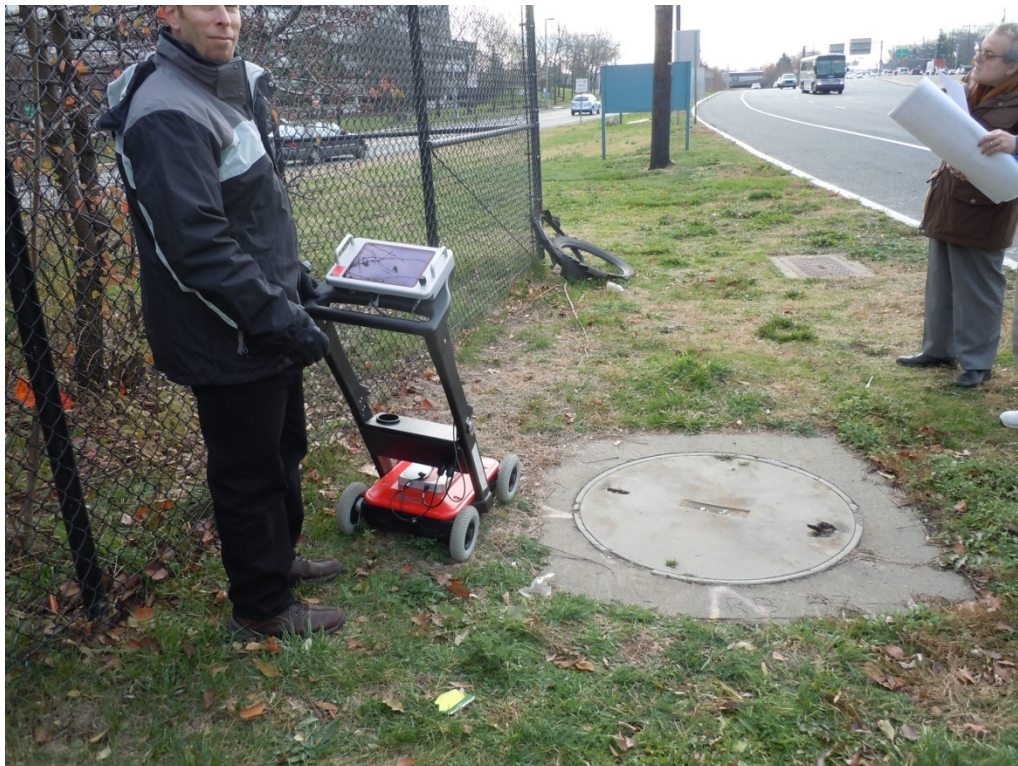
Figure 2 – Mala GPR and junction box
