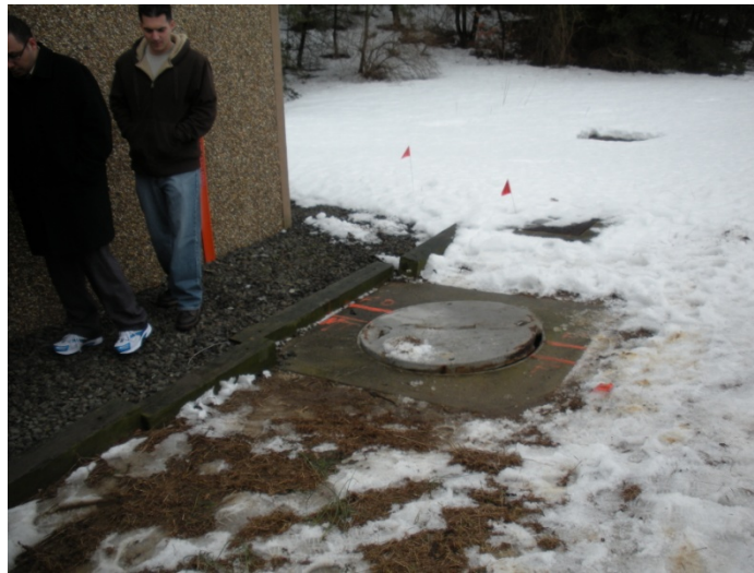
Figure 1: View of site and manhole that provides access to fiber optic conduits. Orange lines indicate the path of two conduits entering and exiting the manhole.
