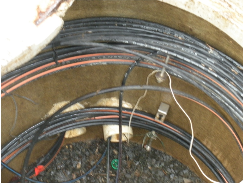
Figure 3: Closer view of conduits on one side. White wire entering one of the conduits is a trace wire. A small transmitter was connected to this wire to generate a signal that could be detected through the earth.
