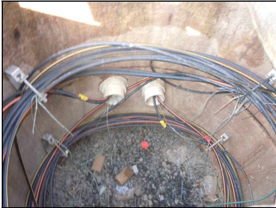
Figure 3b – Inside junction box – right side looking toward road.
