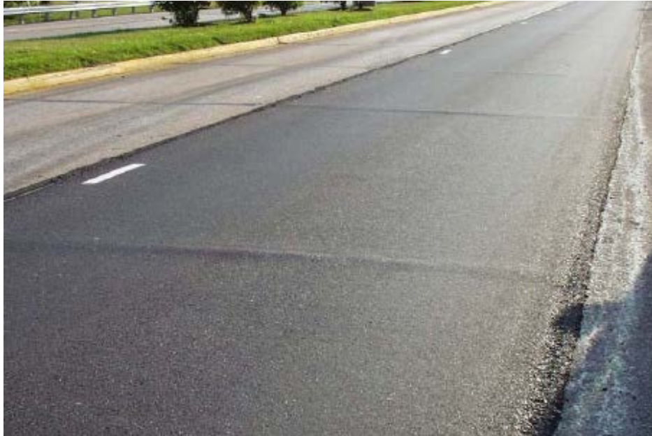
Figure 9. Transverse “Bumps” in the Areas of Rubberized Joint Sealant
