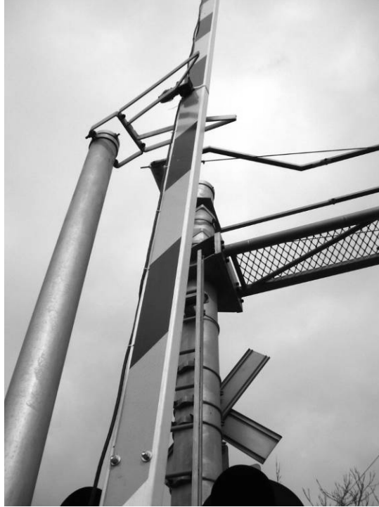
Figure 12. Wind bracket, wind bracket mast, and crossing gate arm at the Broad Street crossing on the NJCL
