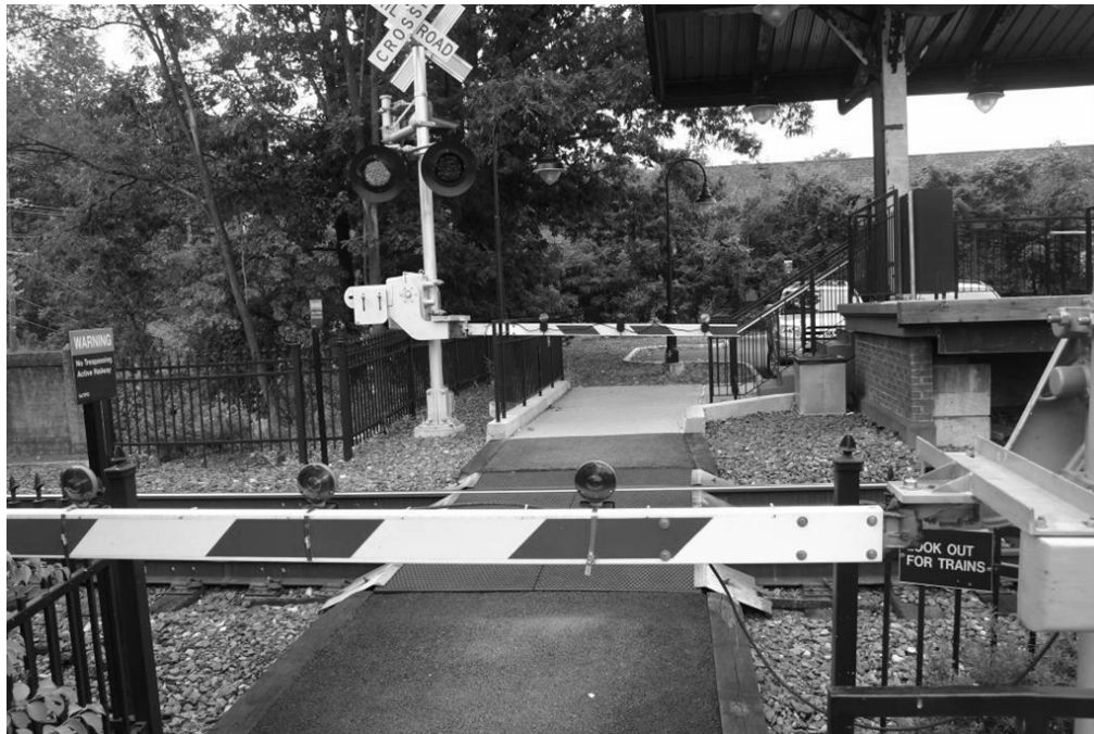
Figure 11. Pedestrian crossing gate arm with typical configuration of flashing lights
