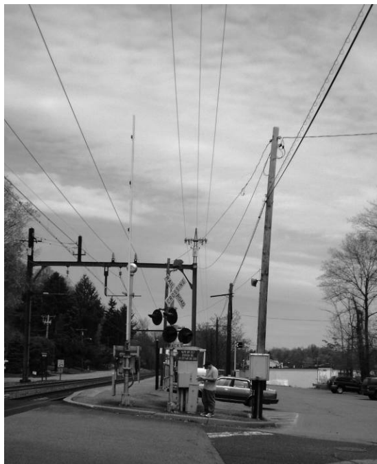
Figure 37. Eastern crossing gate
