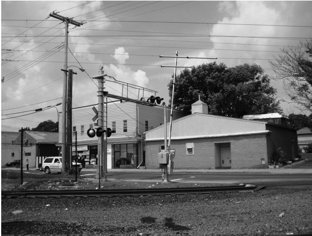
Figure 16. Insulated power lines at the Westwood Ave. crossing on the NJCL
