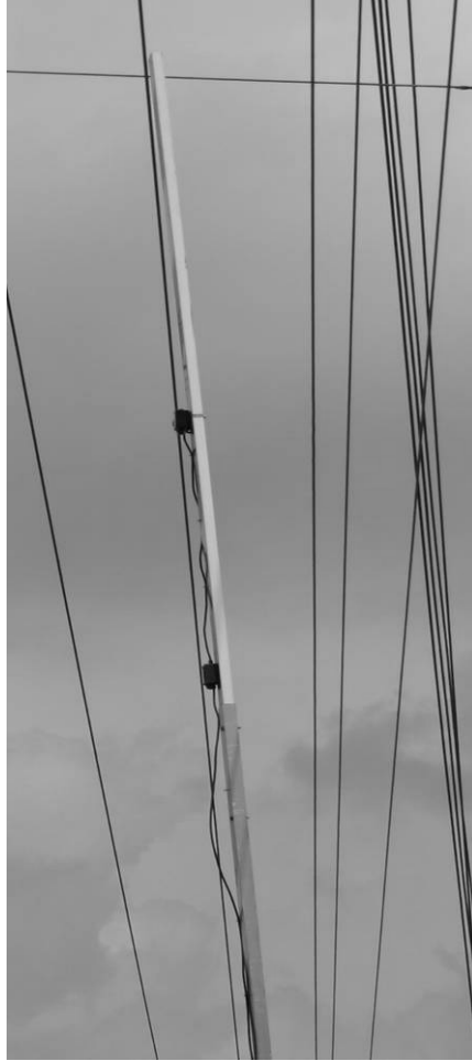
Figure 32. Wires for flashing lights on NW gate arm
