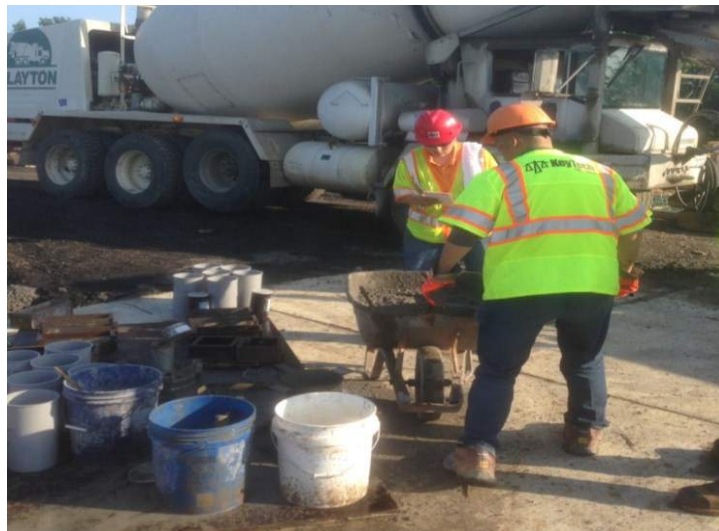
Figure 12. Quality Control Professionals Transporting Fresh Concrete for Slump and Air Pressure Testing
