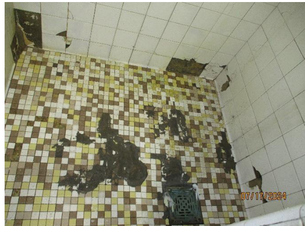
Shower floor in a GSCF General Population housing unit. Photograph by Office of the Corrections Ombudsperson, July 17, 2024.
