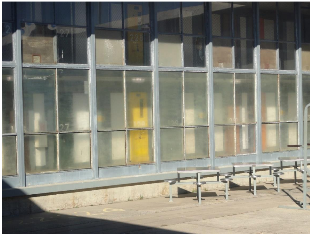
View of Bayside State Prison housing unit from the interior courtyard. Photograph by Office of the Corrections Ombudsperson, January 21 st , 2026.
