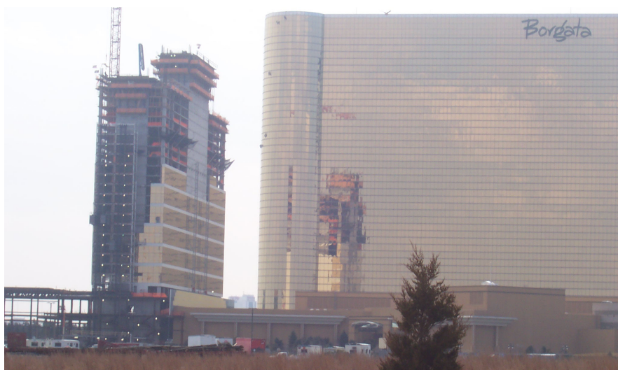
Borgata expansion in Atlantic City. Photographed by Robert Brock, Department of Community Affairs.
