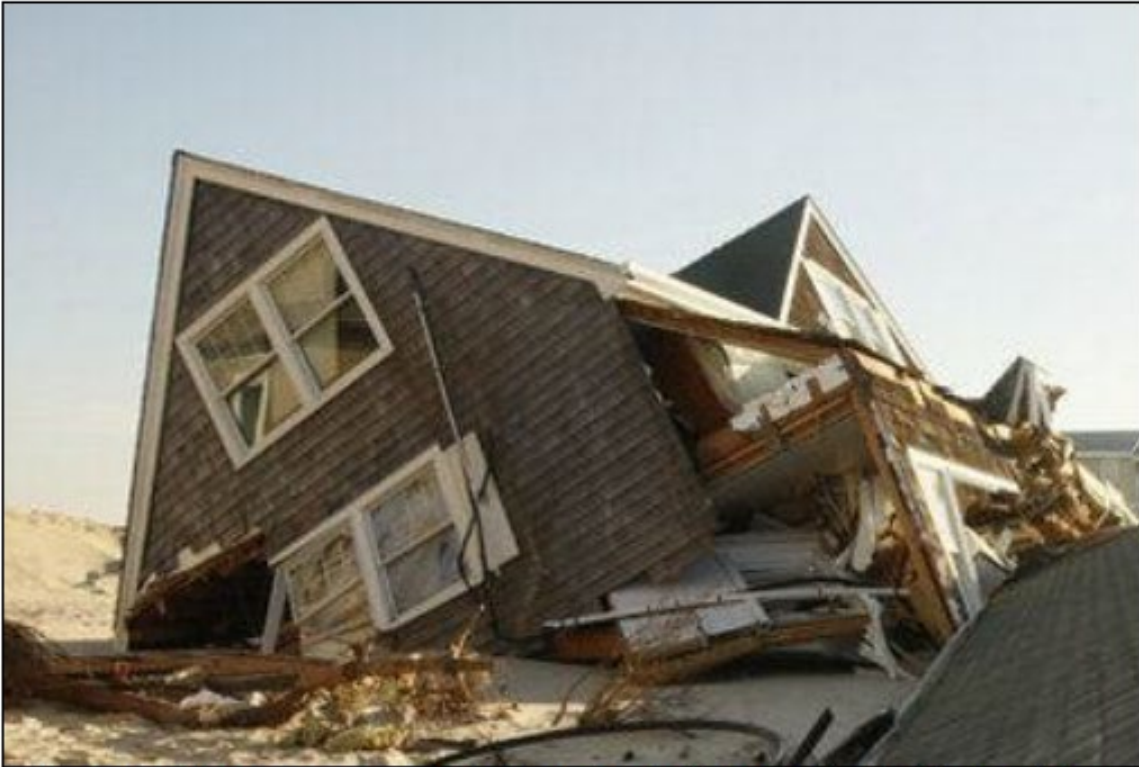
Image #7: The above example photo illustrates a building that is off of its foundation.
