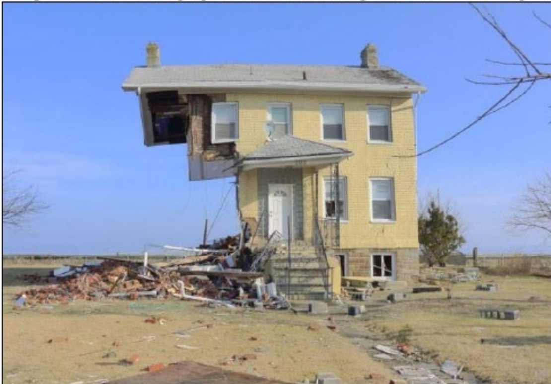
Image #6: The above example photo illustrates a building that is missing one or more complete elevations.
