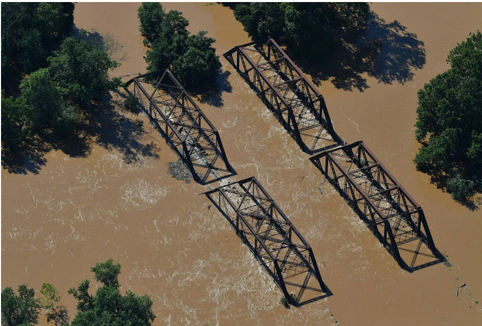
Figure 5: Bridge in Somerset County Inundated by Floodwaters
