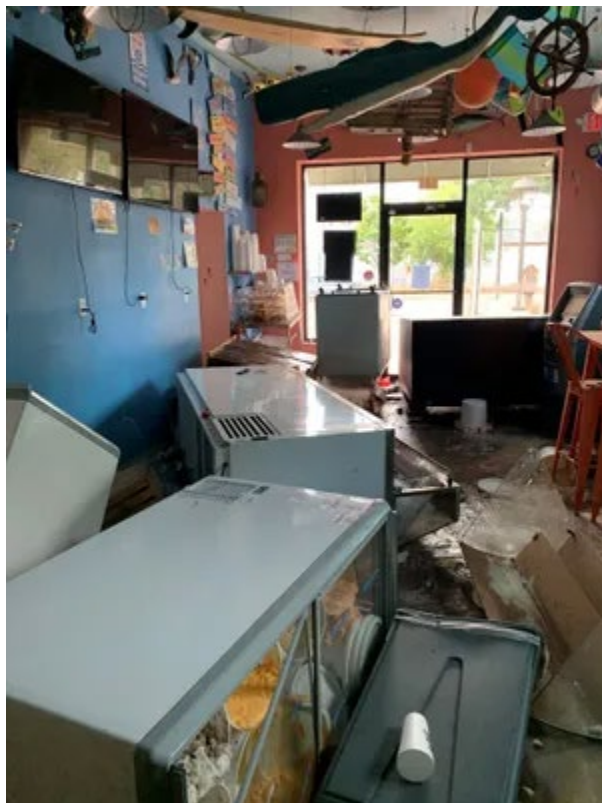
Figure 9: Flood Aftermath at Summer Ville Ice Cream Shop in Somerville, NJ
