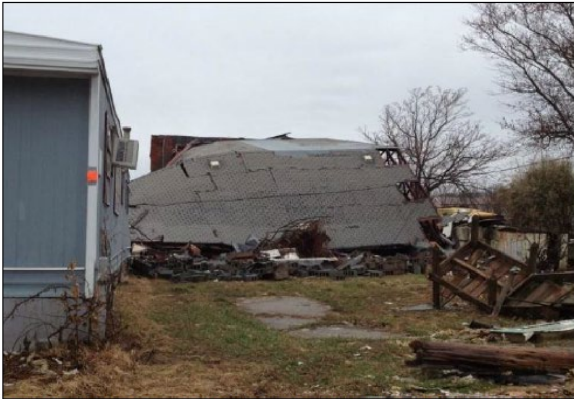
Image #5: The above example photo illustrates a building where the roof has collapsed.
