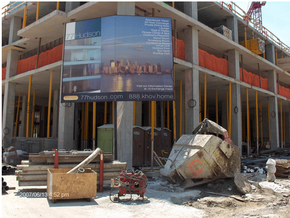
Construction at 77 Hudson Street. Photo by Drake Rizzo and Charles Pierson, Jr., N.J. Department of Community Affairs.
