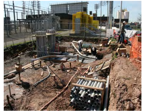
Passaic Valley Sewerage Commission Electrical Substation
