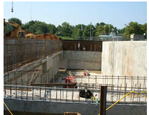
Township of Middletown Sanitary Authority Aeration Digester
