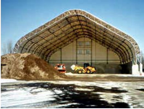
This three sided storage structure does not comply with the permit minimum standard.
