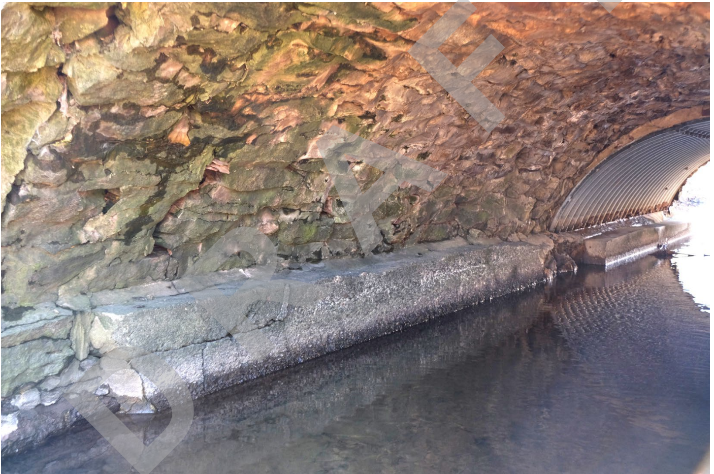
Photo 7: View showing the south half of the barrel vault with the 1938 corrugated metal and concrete barrel vault on the far end.
