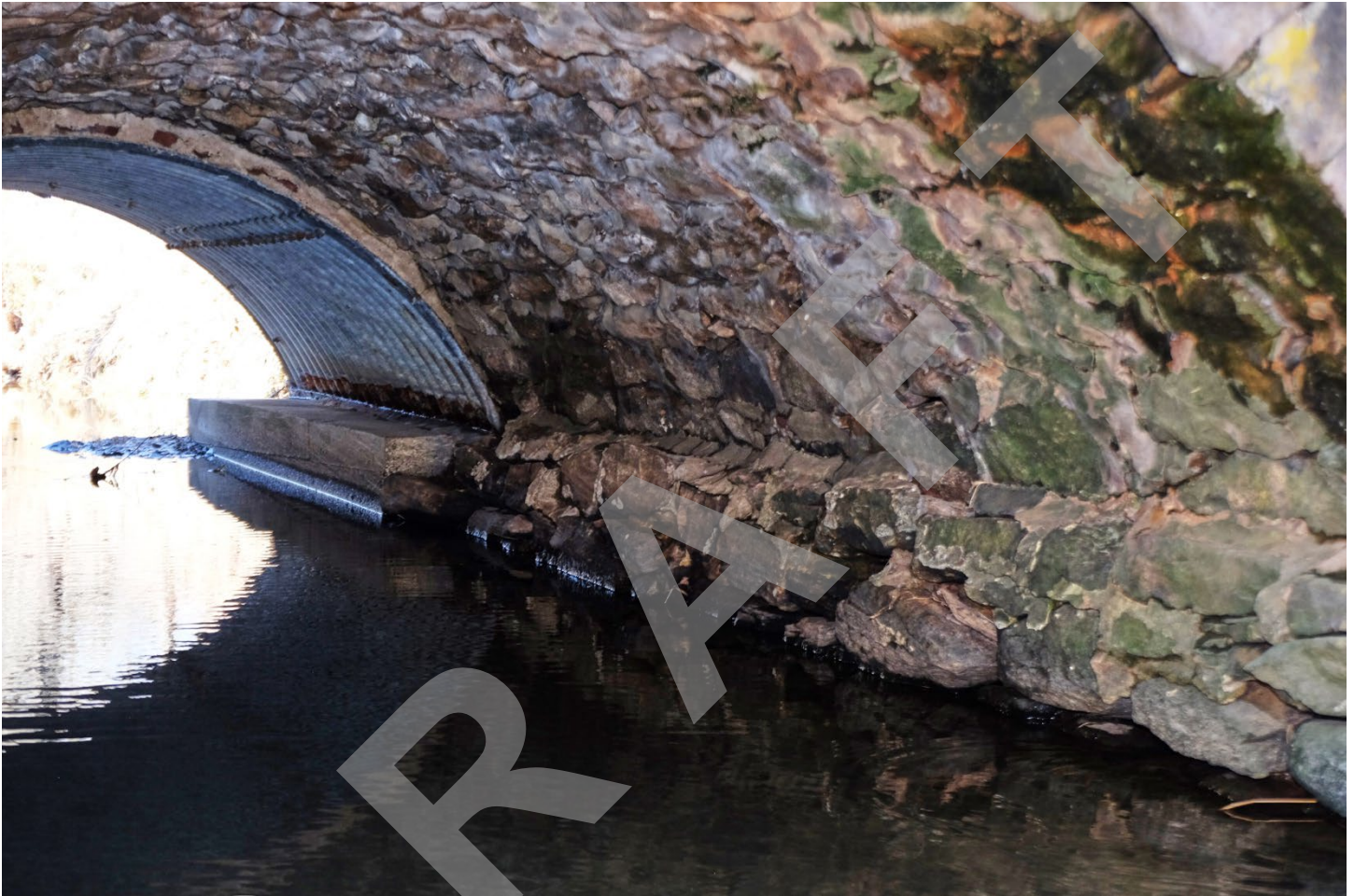
Photo 8: View showing the north half of the barrel vault with the 1938 corrugated metal and concrete barrel vault on the far end.
