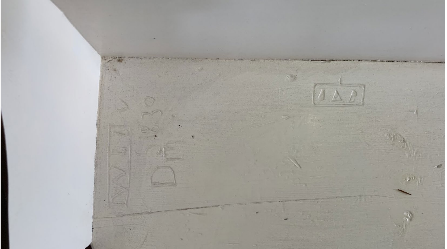
Photo #23: Interior. Second floor, photo of graffiti carved into pew. Includes carved letters and "1830".
