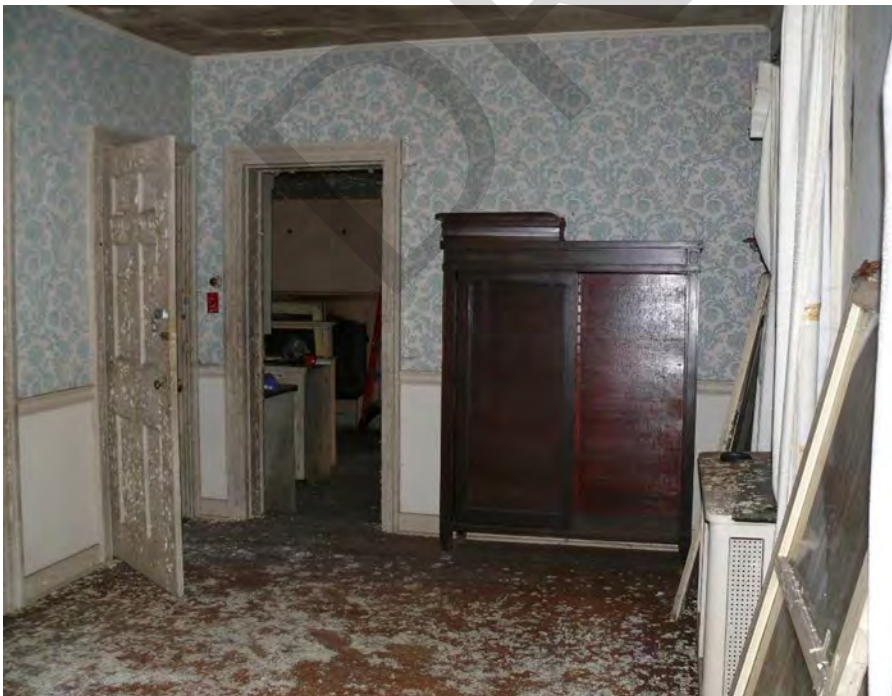
Photo 0016: View of the Dining Room towards the connection with the c.1825 west wing; camera facing west.
