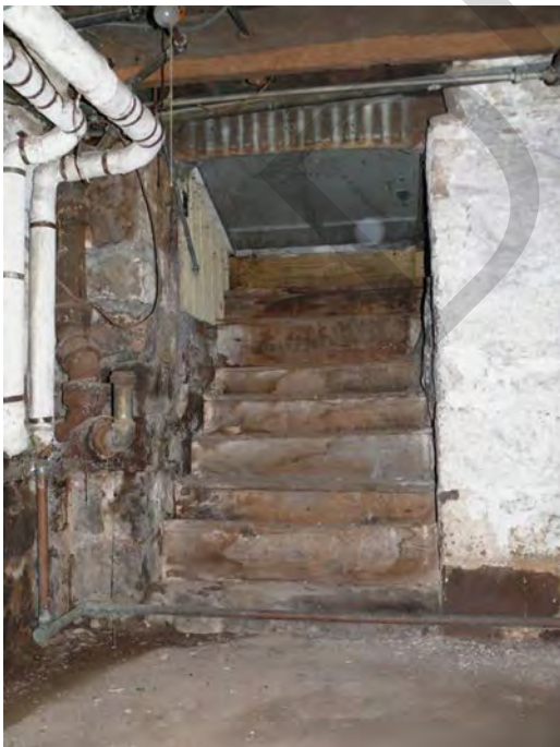
Photo 0010: View of the bulkhead stair at the south end of the west basement wall of the c.1840 east section; camera facing west.
