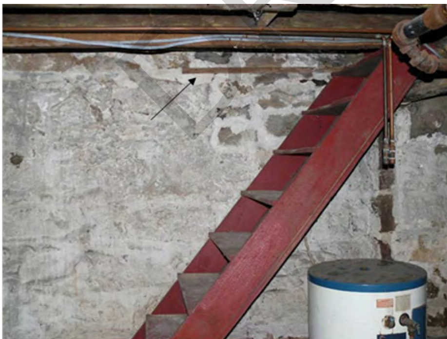
Photo 0012: View of a wood lintel in the west basement wall, which is possible evidence that an opening existing between this basement that of the west wing.
