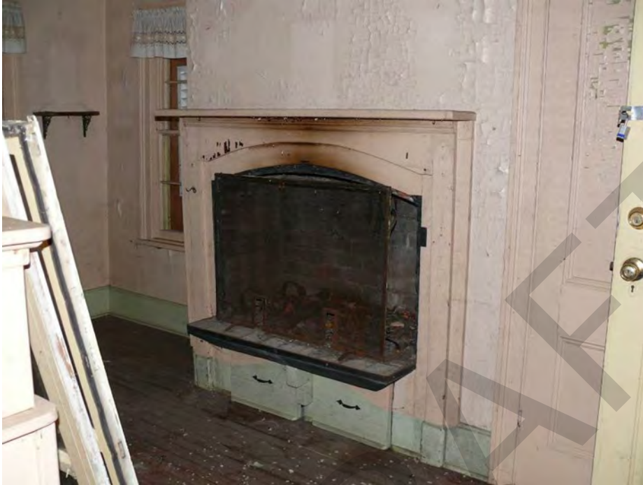
Photo 0017: View of the fireplace at the west wall of the Kitchen; camera facing southwest.
