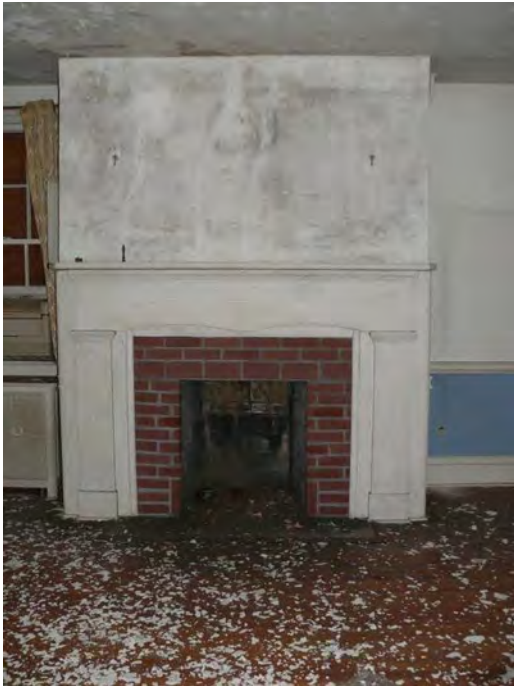
Photo 0015: View of the fireplace at the east wall of the Parlor, which was likely altered during the early-twentieth century; camera facing east.
