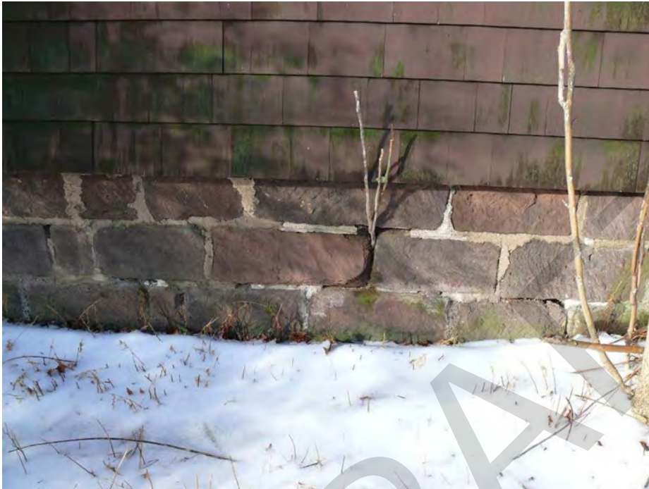
Photo 0003: View of the original ashlar brownstone foundation at the east elevation of the c.1840 east section; camera facing west.
