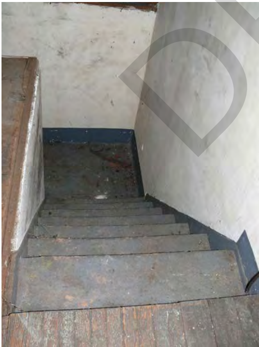
Photo 0022: View of the attic staircase showing plaster wall finishes, wood steps, and plain wood stringer; camera facing south.
