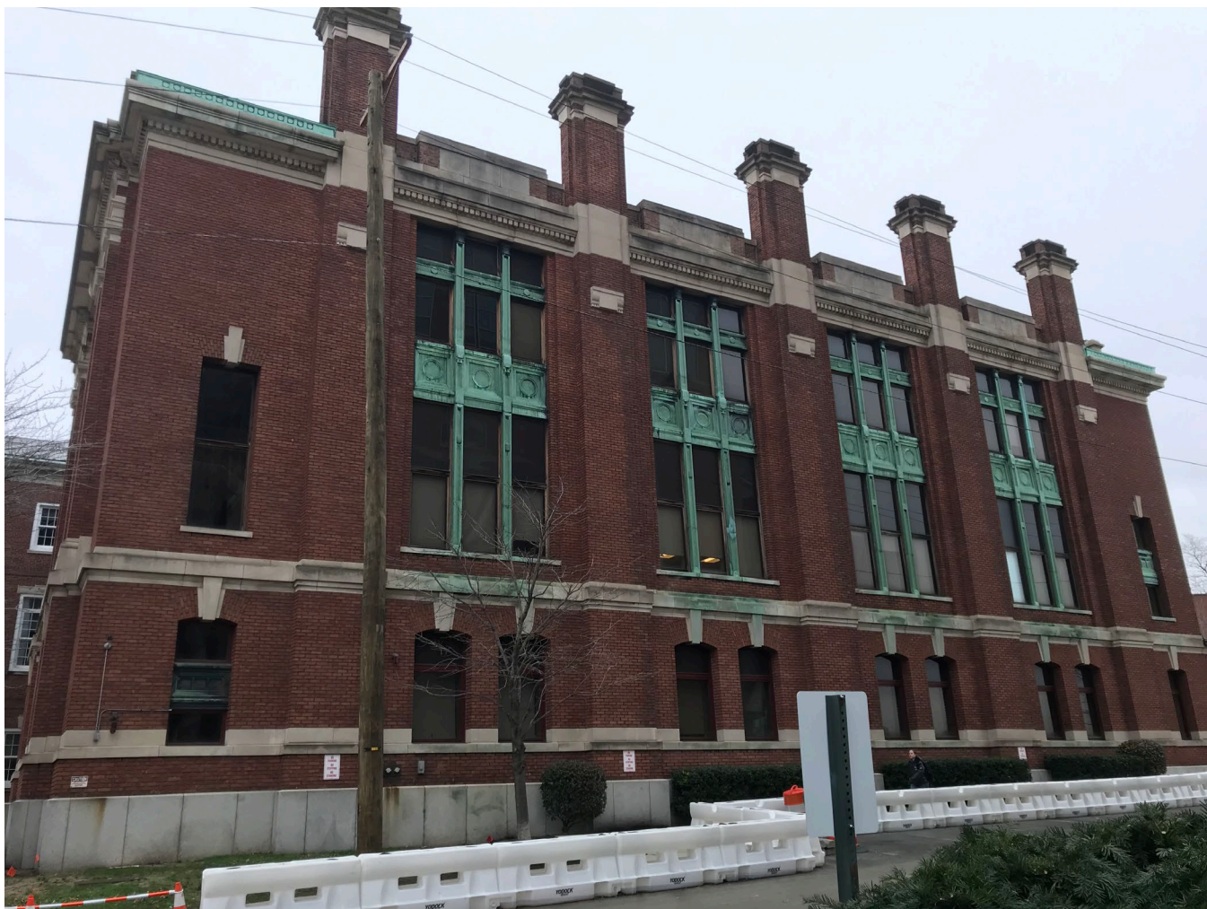
Photo 5. Morton Memorial Laboratory of Chemistry, south elevation. Stevens Institute of Technology, Hoboken (Hudson County), NJ. (Meredith Arms Bzdak, 13 December 2019.)
