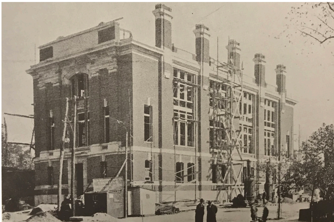
Figure 10. Morton Memorial under construction, 1905 (Archives and Special Collections, Stevens Institute of Technology).
