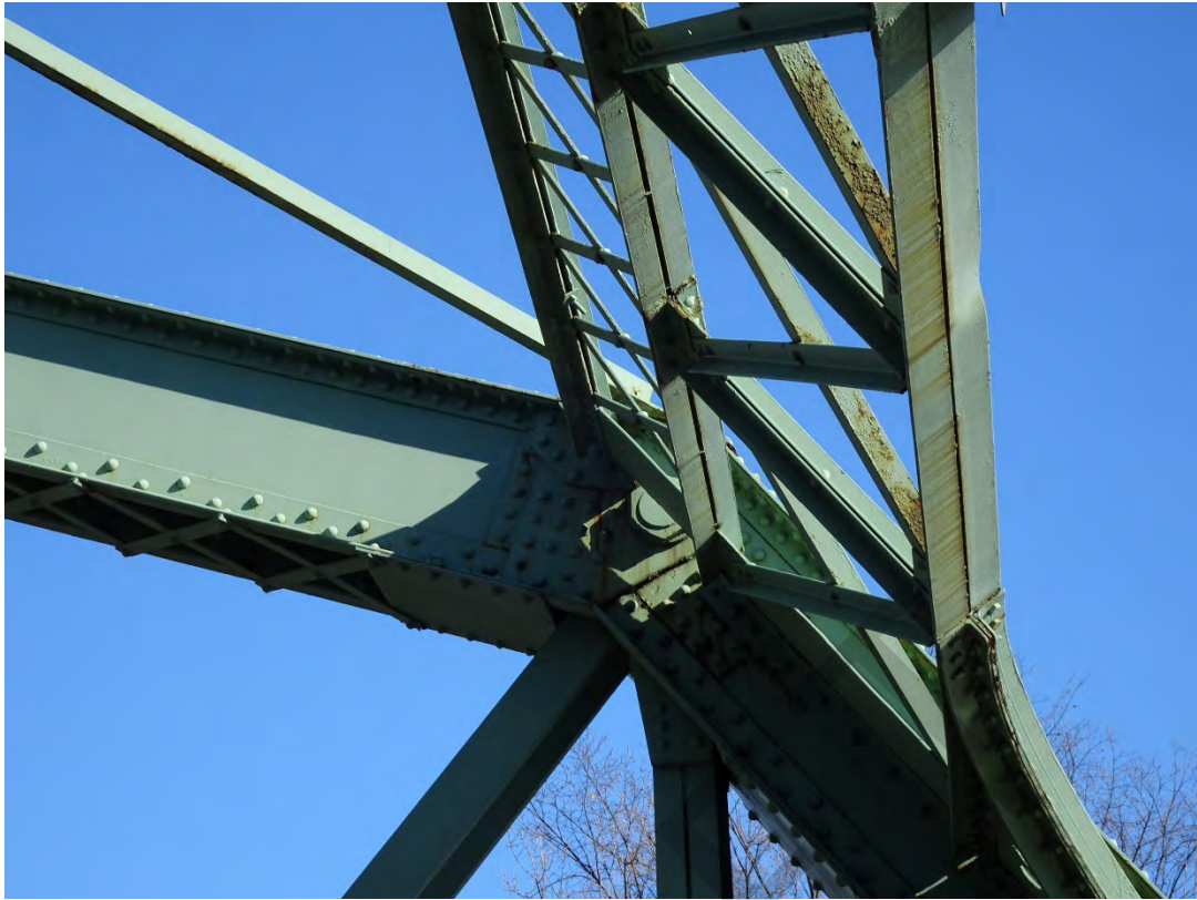
Arch Street Bridge over the Passaic River, City of Paterson, Passaic County Photo #9
