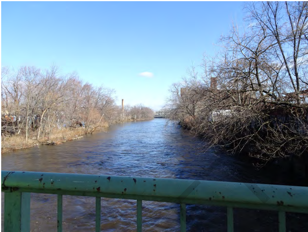
Arch Street Bridge over the Passaic River, City of Paterson, Passaic County Photo #14
