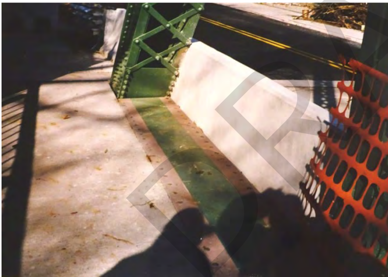
Figures 14, 15. View of the bridge in 1998 shortly after its rehabilitation. Top: Roadway deck looking northwest, showing new concrete and the addition of jersey barriers, Bottom: Detail of new cover plates between pedestrian walkway and the newly installed jersey barriers.
