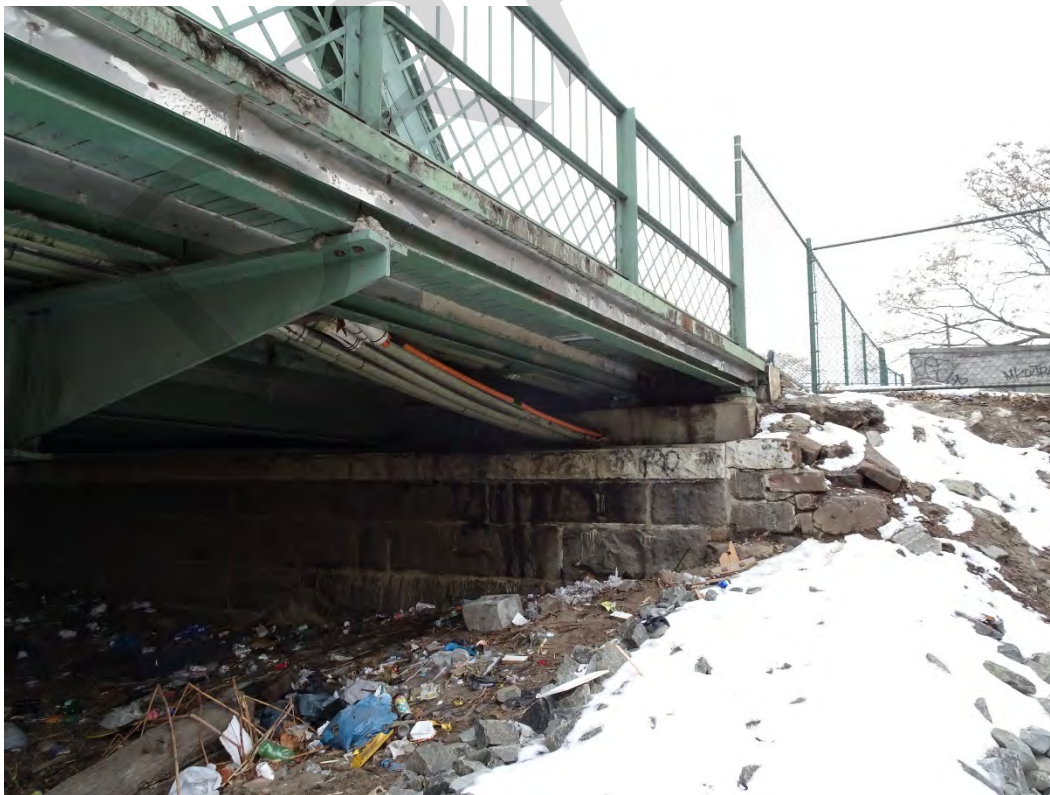
Arch Street Bridge over the Passaic River, City of Paterson, Passaic County Photo #4
