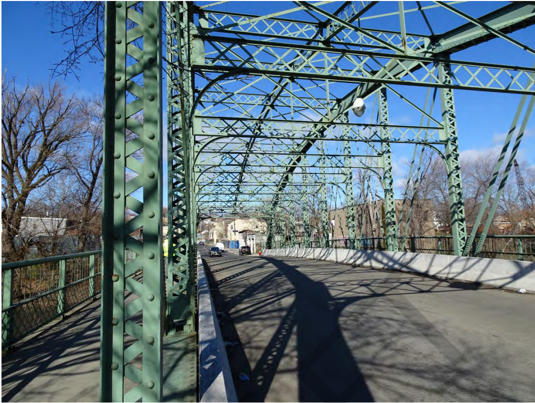
Arch Street Bridge over the Passaic River, City of Paterson, Passaic County Photo #12
