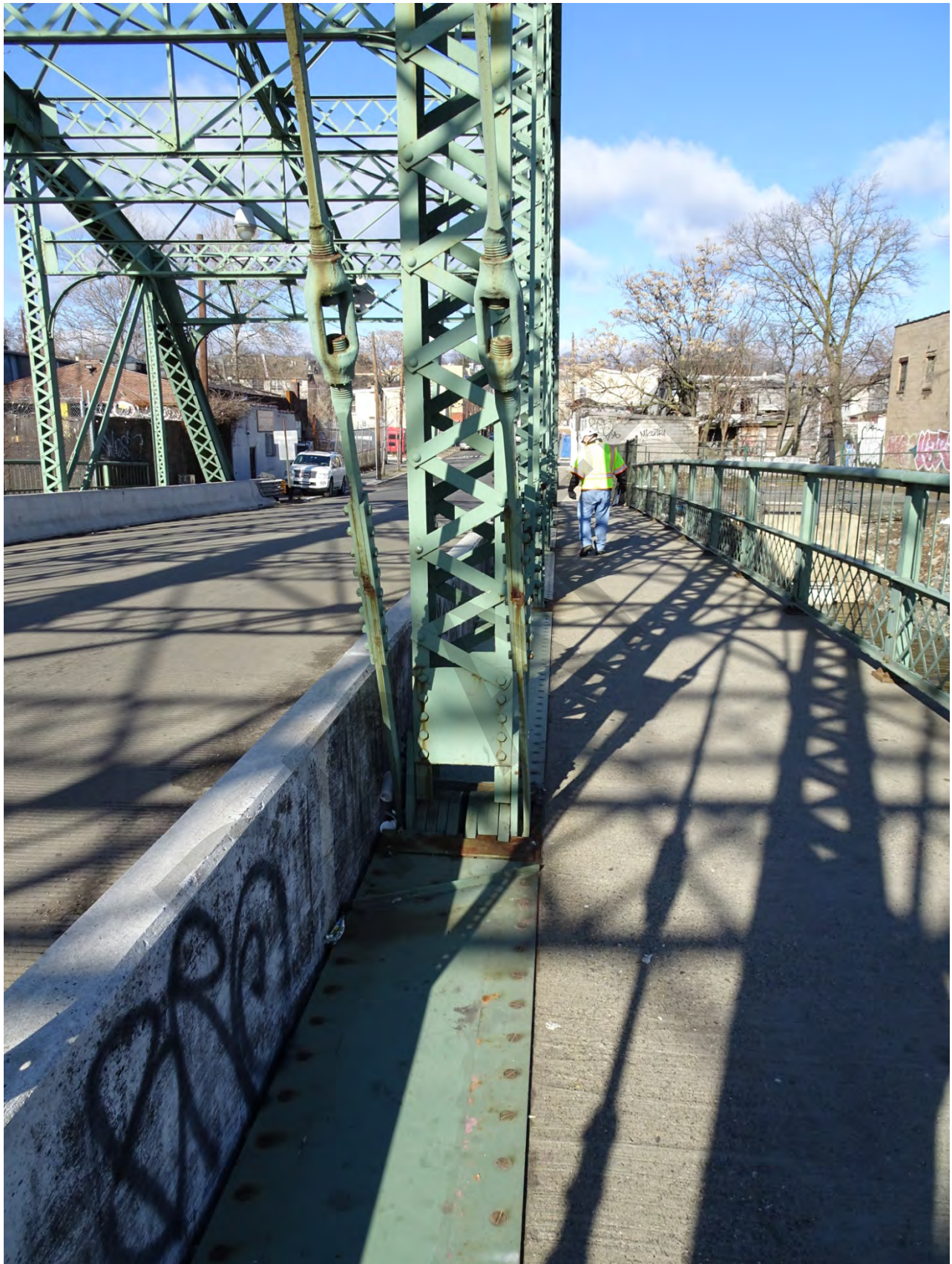
Arch Street Bridge over the Passaic River, City of Paterson, Passaic County Photo #11
