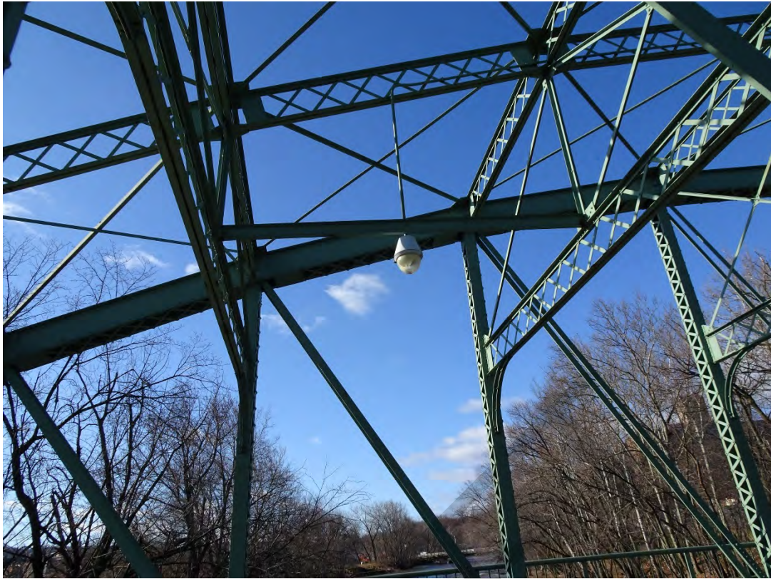
Arch Street Bridge over the Passaic River, City of Paterson, Passaic County Photo #7
