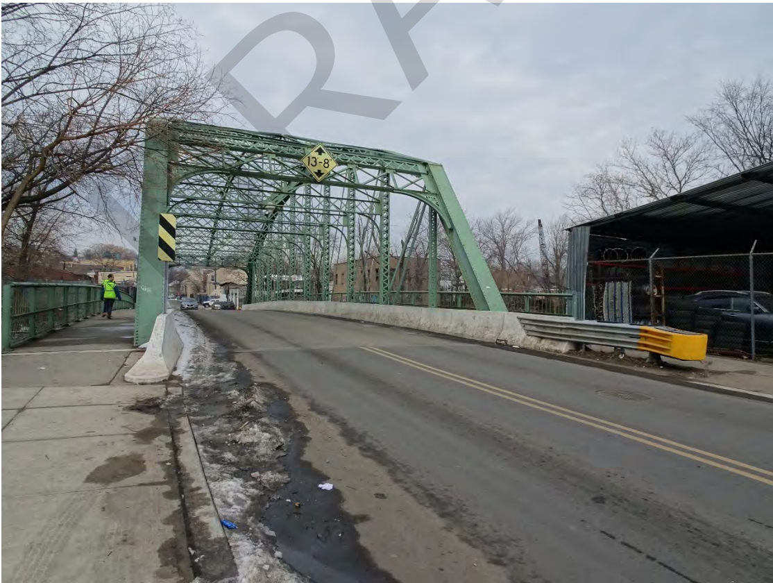
Arch Street Bridge over the Passaic River, City of Paterson, Passaic County Photo #2
