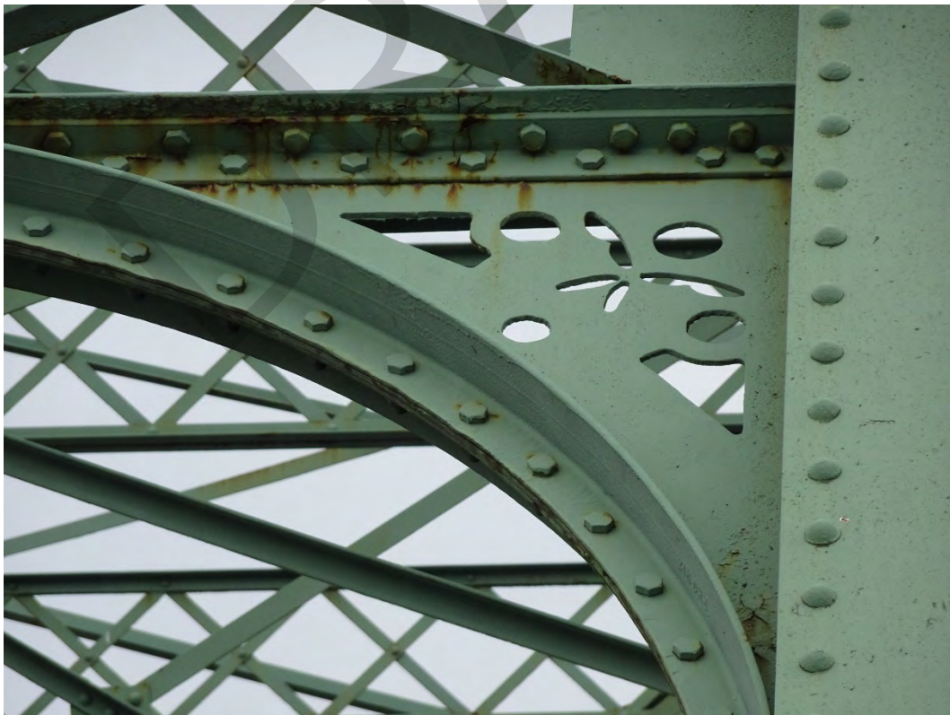
Arch Street Bridge over the Passaic River, City of Paterson, Passaic County Photo #8
