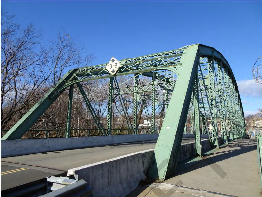
Arch Street Bridge over the Passaic River, City of Paterson, Passaic County Photo #1
