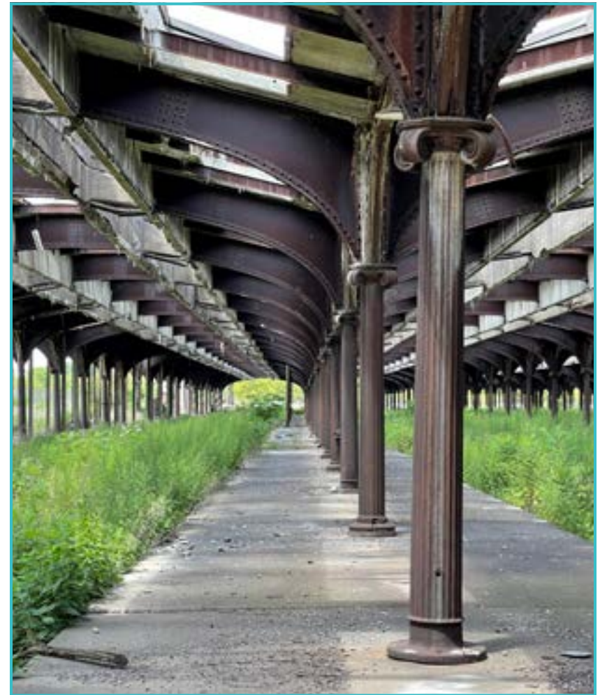
Central Railroad of New Jersey (CRRNJ) Train Shed at Liberty State Park, Jersey City, Hudson County.
