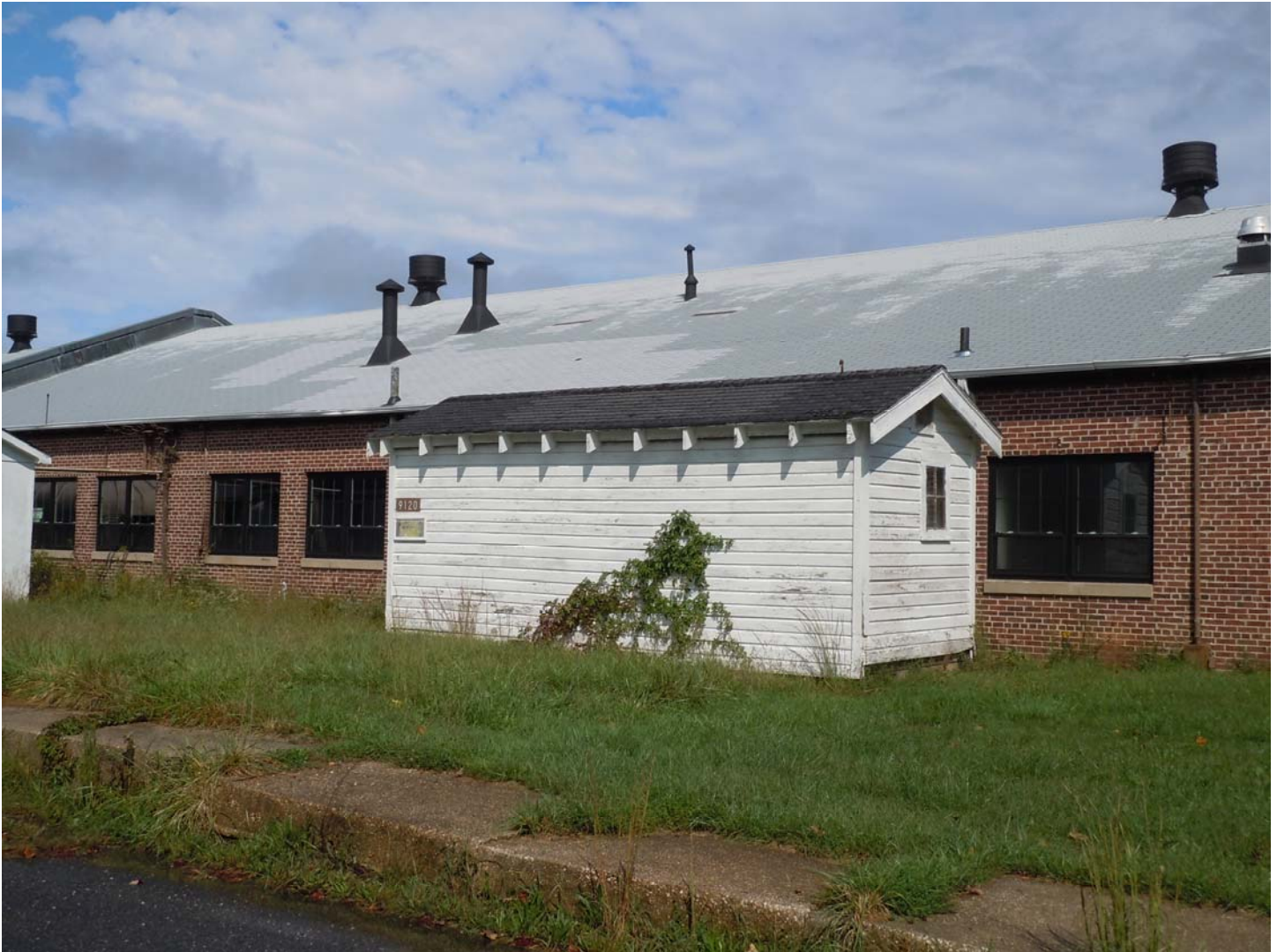
Photograph #20 Gas Cylinder Storage Shed, #9120 (1945), west and south elevations. Robie S. Lange, September 29, 2011
