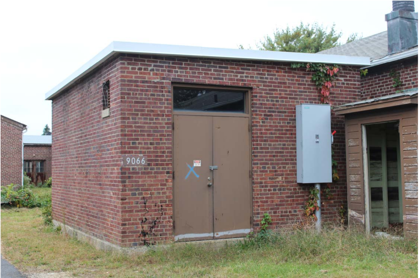
Photograph #18 Transformer Vault, #9066 (1941), east and north elevations. Robert Perricelli, October 12, 2011
