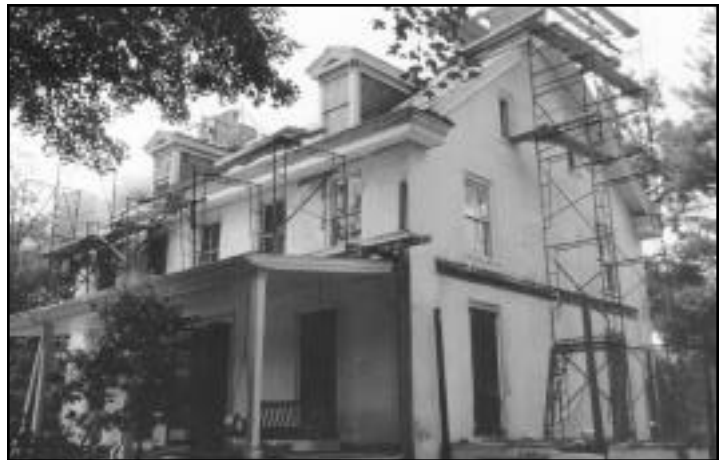
Below: South facade after demolition of kitchen and wrap-around porch – new slate roof being installed.
