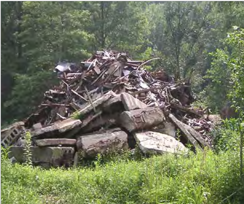
Selective demolition can offer the opportunity of restoring a site to its natural condition and promote water absorption.
