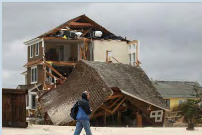
Criteria 5: This residence in Mantoloking, Ocean County is split or sheared. (Photography courtesy of the NJ HPO.)
