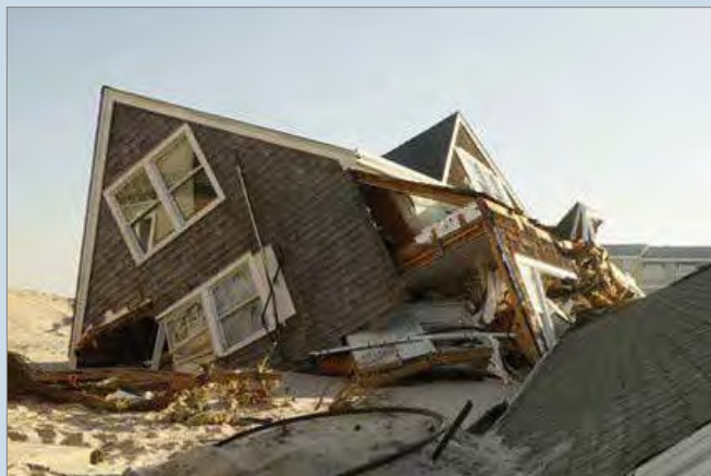
Criteria 4: More than 50% of this residence in Mantoloking, Ocean County is off of its foundation. (Photography courtesy of the NJ HPO.)
