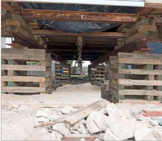
All systems must be disconnected prior to lifting the building off of its foundation.
