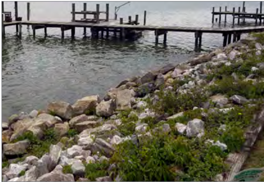
Rip-rap represents a means of structural shoreline protection.
