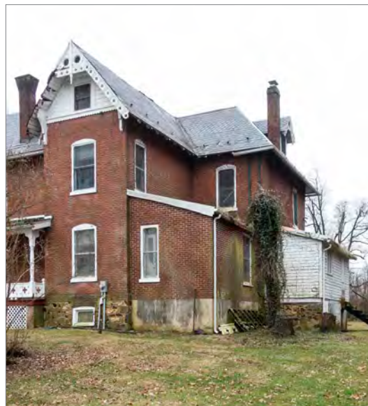
A poorly maintained building is less likely to withstand flood damage than a well maintained building. If the structural system is compromised, it will be more difficult and more costly to elevate or relocate.
