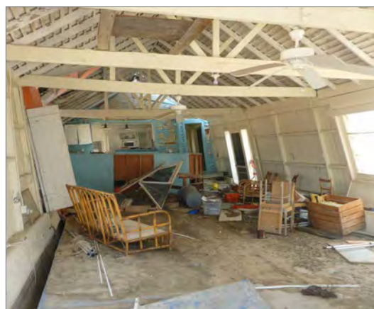
If the level of damage is such that the cost to restore the building to its pre-damaged condition it will likely meet the definition of “substantial damage” in a municipal floodplain ordinance. (Photograph courtesy of the NJ HPO.)
