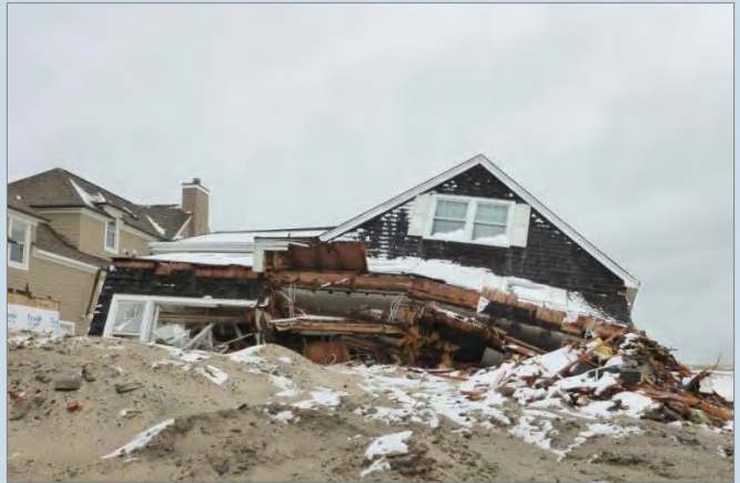
Criteria B: This residence in Mantoloking has pancaked, with the lower floors resting on the ground below. (Photography courtesy of the NJ HPO.)
