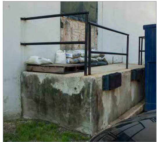
Sandbags can provide temporary protection at doorways. However, they substantial available materials, onsite trained personnel to properly stack bags, and appropriate disposal methods if contaminated by floodwater
