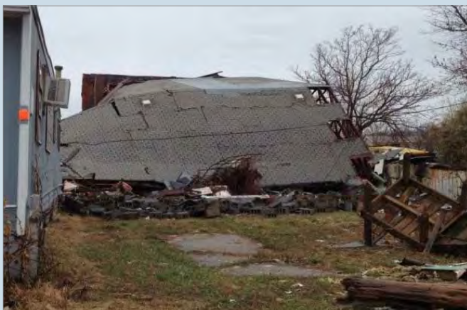
Criteria 2: The roof has collapsed on this Highlands, Monmouth County building. It is also likely that it meets Criteria B for pancaking. (Photography courtesy of the NJ HPO.)
