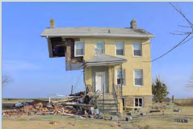
Criteria 3: This Union Beach, Monmouth County residence is missing one or more of its complete elevations. (Photography courtesy of the NJ HPO.)
