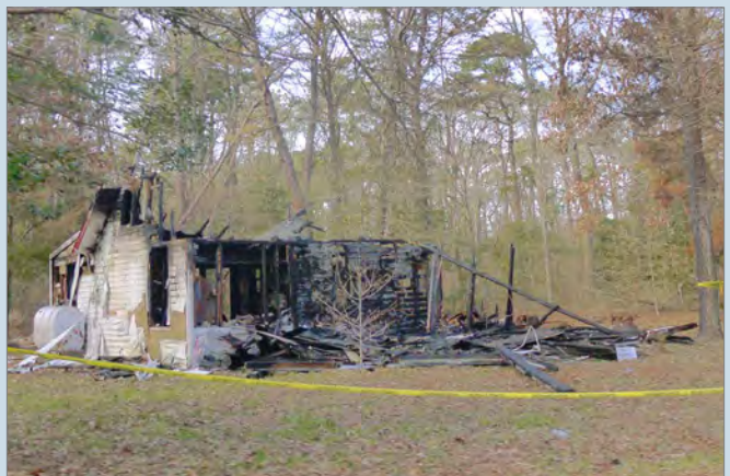
Criteria C: Fire damage has structurally compromised this building in Brick, Ocean County. (Photography courtesy of the NJ HPO.)
