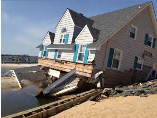
Response includes performing initial inspections of properties to assess building stability and level of damage.
