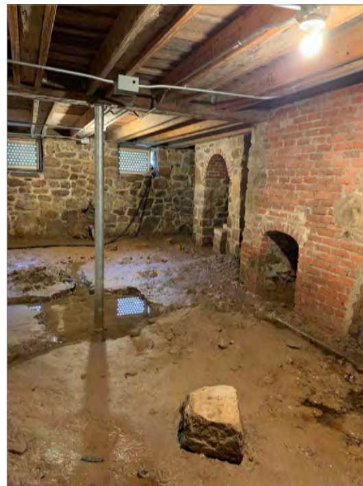
An understanding of building's condition as well as foundation design and materials is necessary to determine flood risk. Basement finishes, such as a basement floor slab, can prevent stormwater or ground water drainage.
