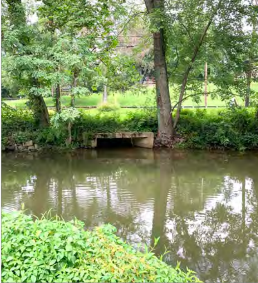
Stormwater runoff from the adjacent roadway discharges directly into the canal.
