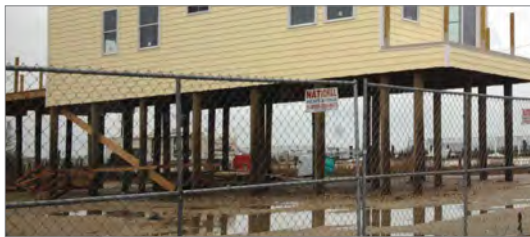
Open piles without screening are generally incompatible with historic buildings. (Photograph courtesy of NJ HPO/FEMA.)
