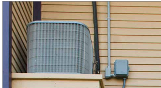
The air conditioner unit is inconspicuously located on a raised platform at the side yard to minimize its visibility from the street.
