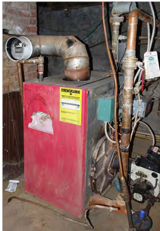
Building systems and equipment are often located in basements where they are highly susceptible to flood damage, necessitating costly replacement.
