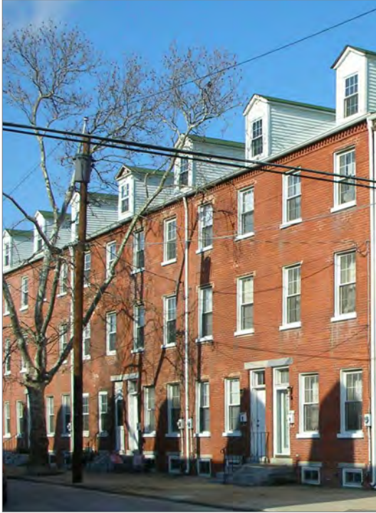
The shared party walls in row houses make them difficult to elevate. However, non-structural elevation in which lower level(s) are abandoned could be a viable mitigation measure. (Refer to page 36.)
