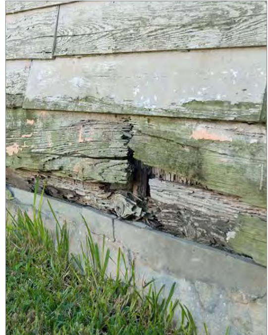
Wood, particularly unpainted wood near the ground, is highly susceptible to damage when exposed to flood water.
