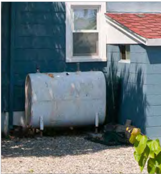
Propane tanks can provide an alternative fuel source however, they should be secured to prevent floatation in a flood event.
