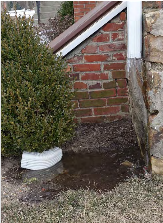
A key component of maintenance to reduce potential flood damage is to ensure that stormwater collected by gutters and downspouts flows away from a building rather than pooling adjacent to the foundation or support systems.
