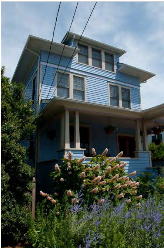
The landscaping at this building is very lush and conceals the foundation.
