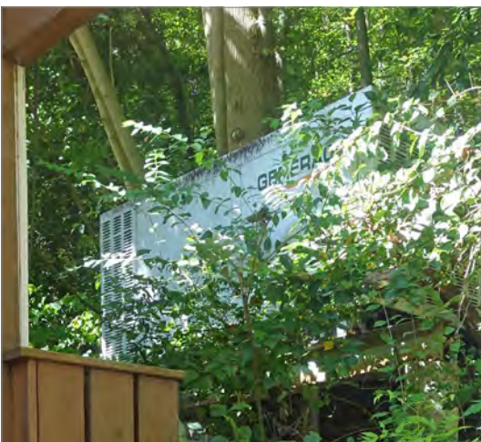
The back-up generator is located up on the hill and concealed by foliage.
