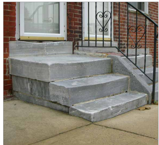
Stone stoops are character-defining features of many row houses and their alteration should be avoided.
