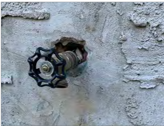
Sealing opening around penetrations such as hose bibs is recommended.
