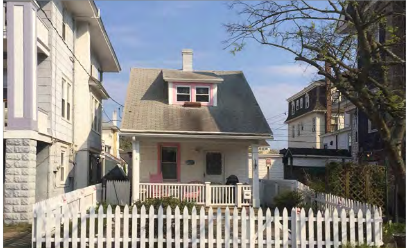
The flood vulnerability for this small cottage is much higher than its elevated neighbors. (Photograph courtesy of NJ HPO/FEMA.)
