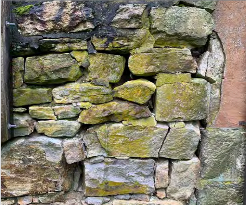
Proper maintenance can impact the flood resilience of materials. Although the stone may be an acceptable flood resistant material, the lack of mortar provides a path for flood water ingress.
