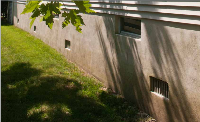
Flood vents, such as those located along the foundation, allow the free passage of water in and out of a closed foundation or building.
