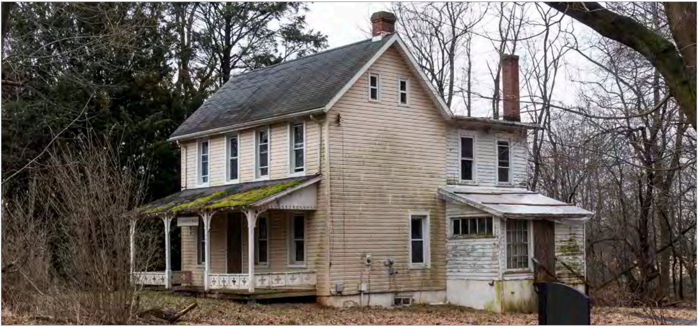
Poorly maintained buildings are more susceptible to damage from flooding and may require stabilization prior to elevation.
