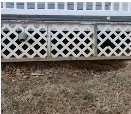
The soil at the base of the porch has eroded and storm water drains towards the building foundation. Regrading to provide storm water drainage away from the building is recommended.
