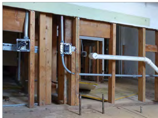
Interior drywall was removed and electrical outlets and plumbing connections were raised following a flood.
